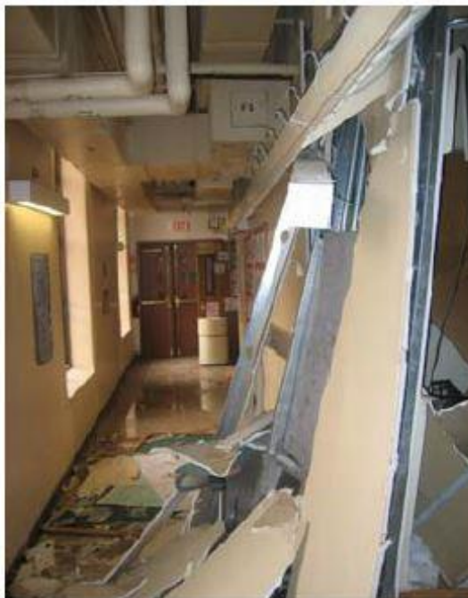
Figure 2 - Hallway Outside Laboratory Showing Explosion Damage
