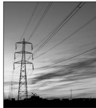
Power lines carry electrical energy safely from the power plant to homes and businesses.
