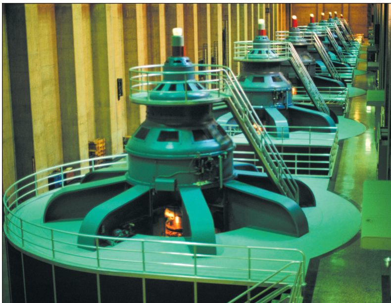
This power plant at the Hoover Dam in Nevada uses the energy from falling water to generate electrical energy.
