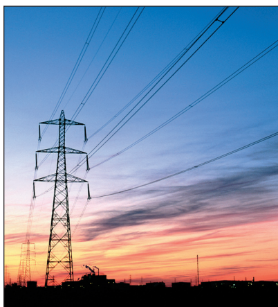
Power lines carry electrical energy safely from the power plant to homes and businesses.
