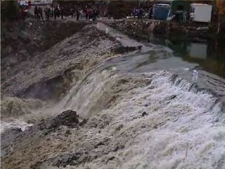
e. Progressive erosion of headcut (12:59)
