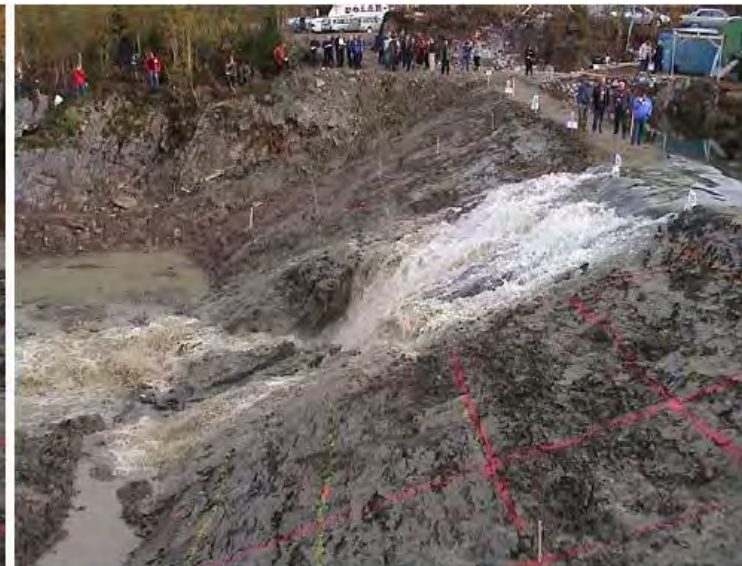
b. Formation of small headcut (12:07) near toe of embankment
