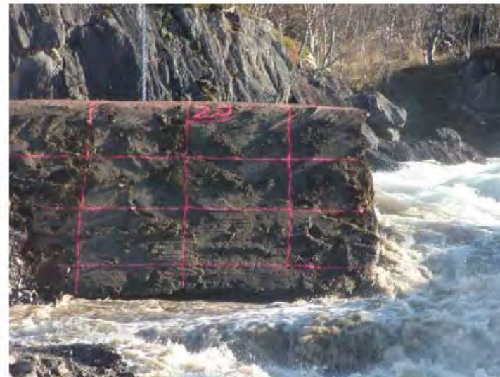
d. Breach sides remain vertical or undercut during the breach formation process
