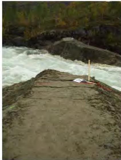
a. Tension crack forming in crest; embankment ends rotating into breach
