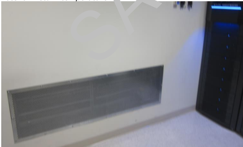
Low wall return to a FM50 unit, located in cold aisle space
