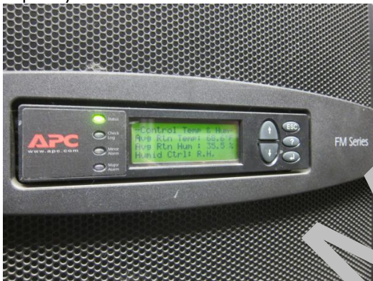
APC FM50M-AKA-ESR Unit control panel, note low return temperature
