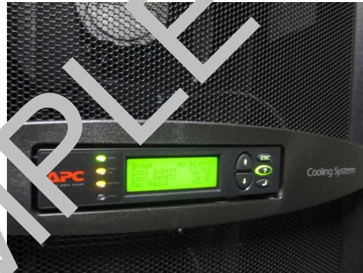
In-row cooler control panel
