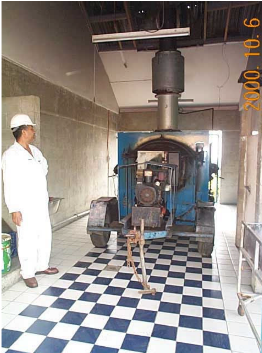
Plate 11: Garbage Being Transferred Direct to a Truck via a Chute
