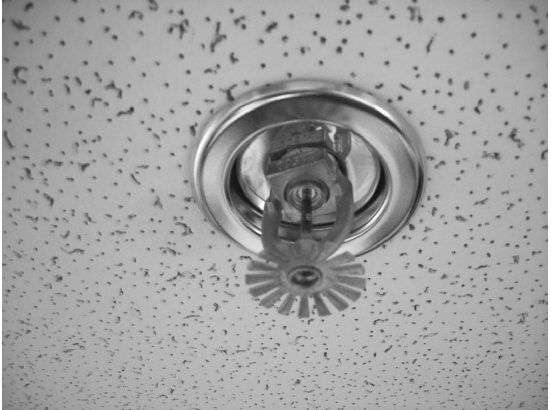
Figure 8-16 Fire sprinkler head
