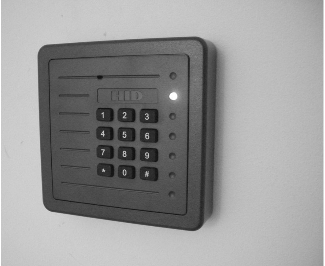
Figure 8-4 Card reader and PIN pad protects sensitive facilities
