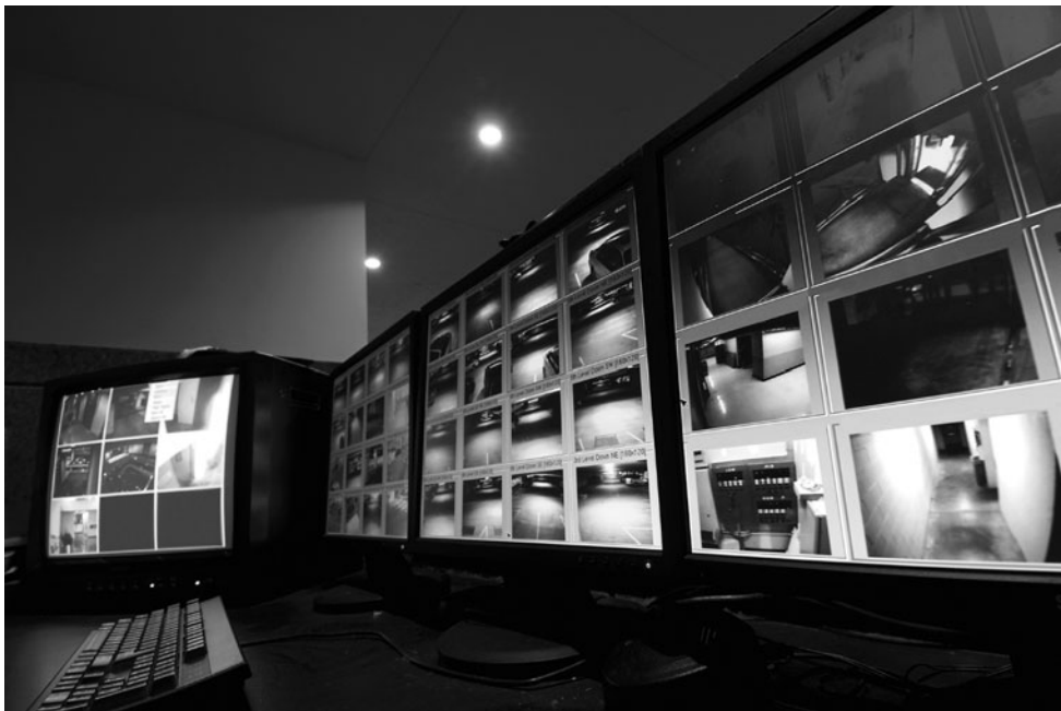
Figure 8-9 Video surveillance monitors
