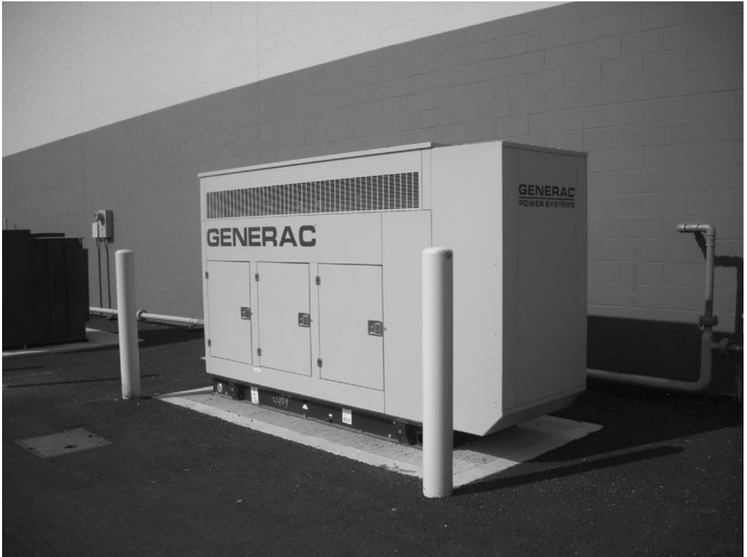
Figure 8-17 Electric generator produces electric power when utility power is unavailable
