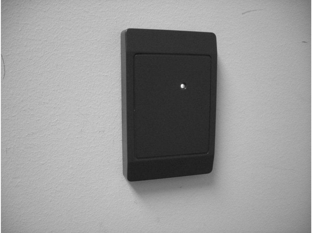
Figure 8-3 Key card reader used to control physical access
