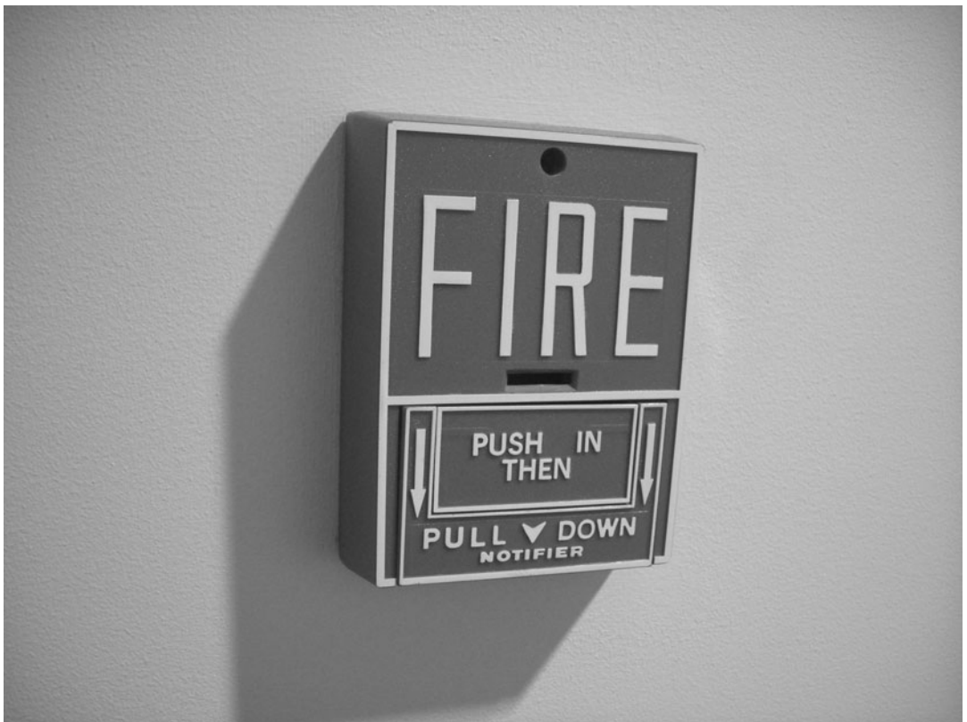
Figure 8-14 Fire alarm manual pull station
