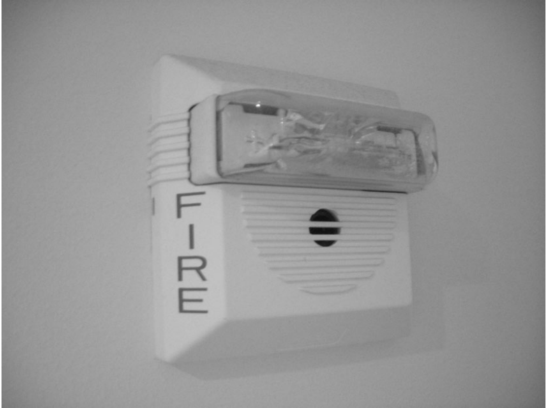
Figure 8-15 Fire alarm annunciator
