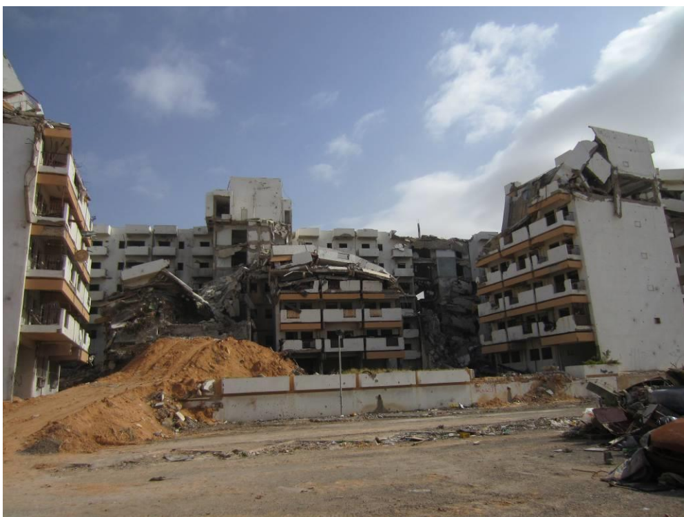
Apartment building struck on 16 September in Sirte © Amnesty International
