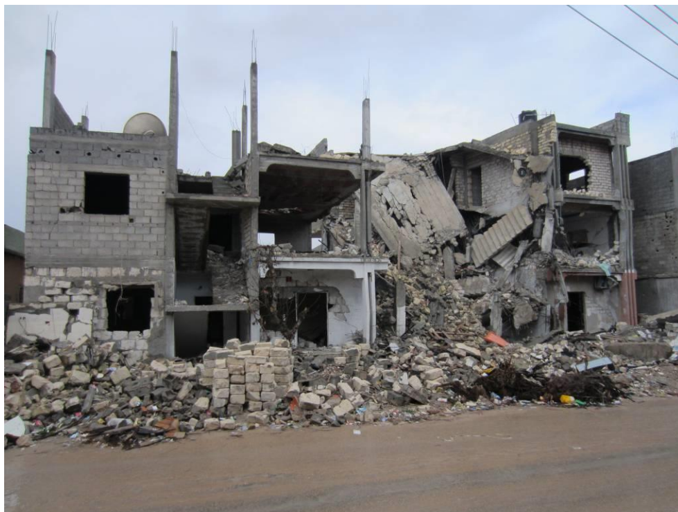
Home of Mukhtar al-Gharari, in the Souq al-Juma'a district of Tripoli, struck on 19 June 2011 © Amnesty International
