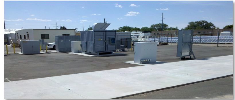
Energy Storage Test Pad (ESTP)
