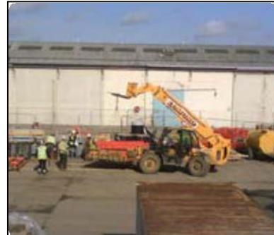
Attachment and load incorrectly positioned
