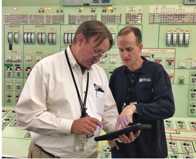
Figure 10. A control room operator and a field operator at Diablo Canyon Power Plant discuss a procedure using the CBP system on the hand-held device.
