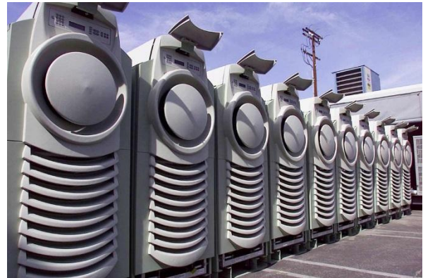
Figure 15: Image of Parallel Capstone Microturbines
