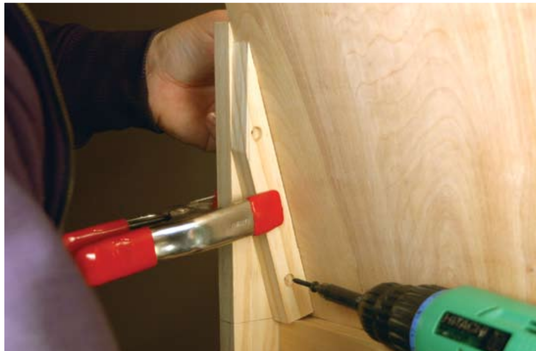
17 Some glue, a spring clamp and a couple of screws (in countersunk holes) added the braces and made the back much stronger.
