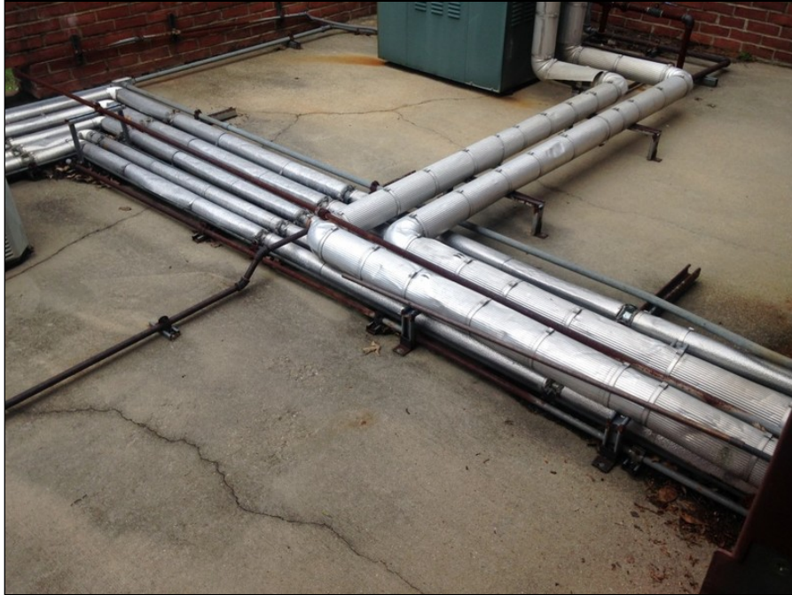
11 - View of exterior piping
