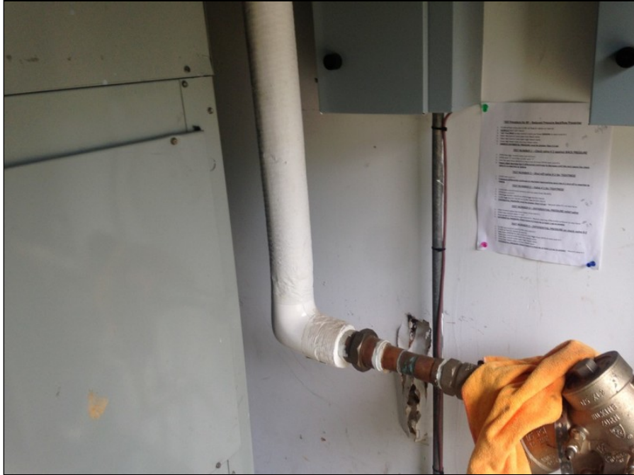
9 - View of piping and wall materials in the mechanical room
