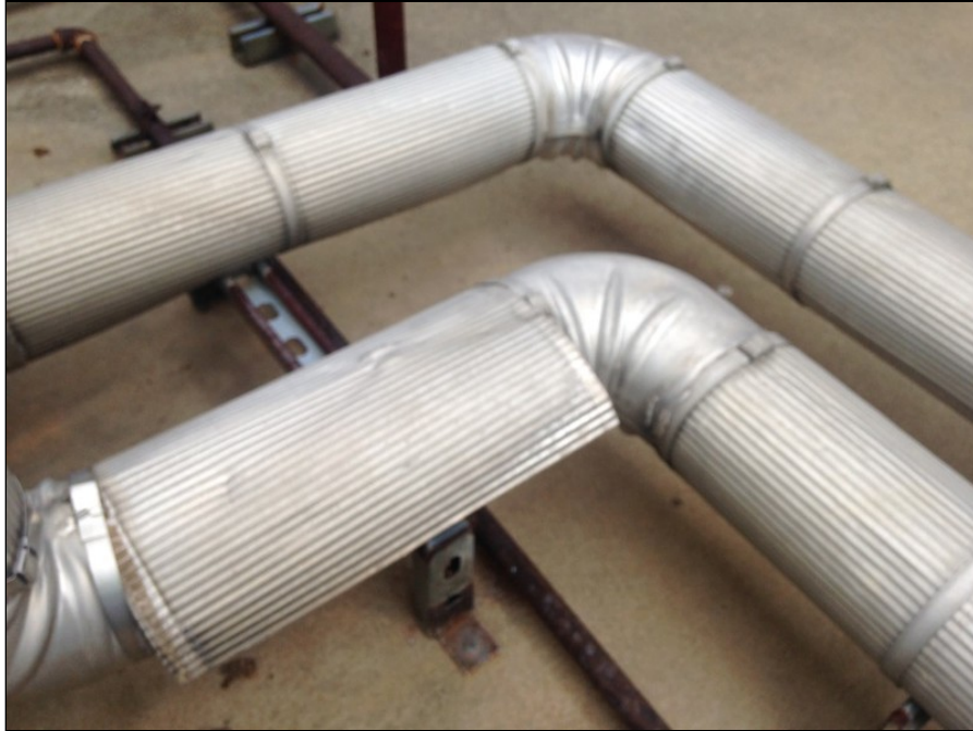
13 - View of exterior piping
