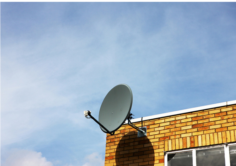
FIGURE 1. PARABOLIC DISH ANTENNA
