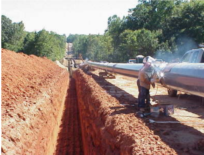
FIGURE 3.3-10 Welding Pipe (Source: Photos courtesy of U.S. Pipeline, Inc. Reproduced with permission.)
