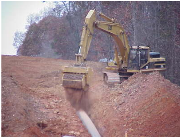
FIGURE 3.3-14 Backfilling Pipeline (Source: Photos courtesy of U.S. Pipeline, Inc. Reproduced with permission.)
