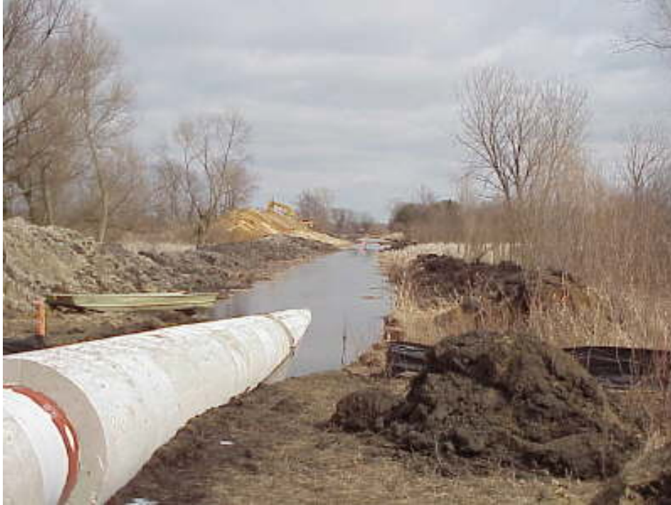
FIGURE 3.3-25 Concrete-Coated Pipe in a Wetland (Source: Photo courtesy of U.S. Pipeline, Inc. Reproduced with permission.)
