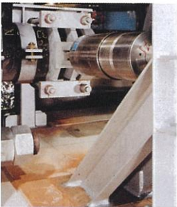
Examples of shock absorber installation in nuclear plants
