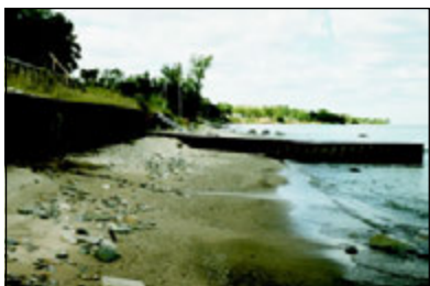
A bulkhead and companion breakwater in Sanilac County, Michigan, on Lake Huron
