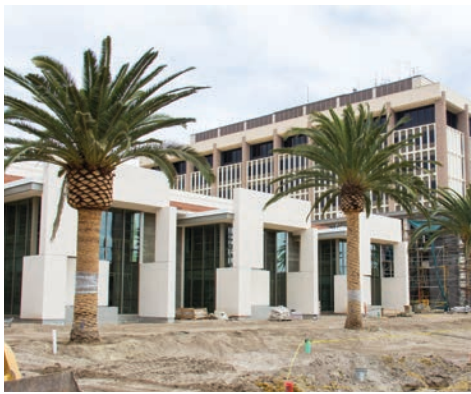
With scaffolding down and new palm trees out front, the Library's three-story addition and two-story renovated building (left) are emerging from their construction cocoon. (Library/Jonathan Rissmeyer)
