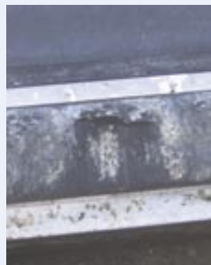
A close up of the damaged hinge
