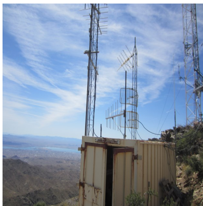
A view of the repeater housing with a look down into Lake Havasu City.
