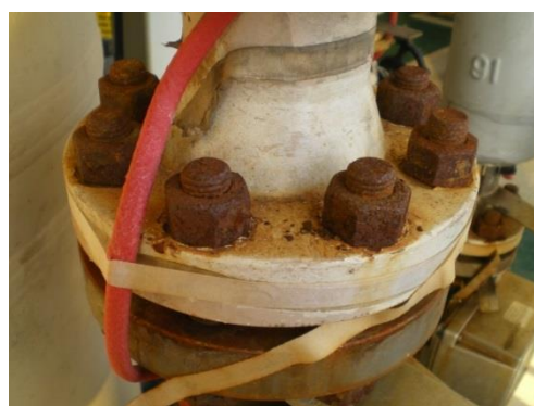
Fig 12 - Bolt corrosion after 18 months offshore North Sea
