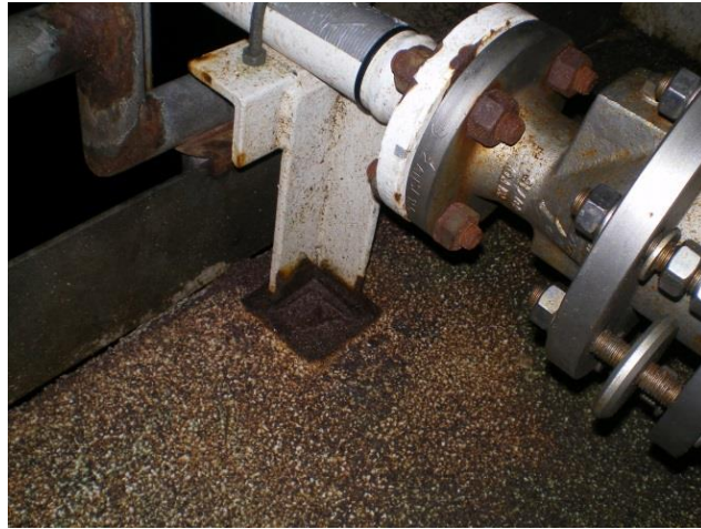
Fig 4 - rusting carbon bolts in stainless substrate
