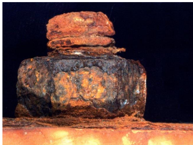
Fig 3 - PTFE/zinc coated bolt failure after 18 months in the splash zone
