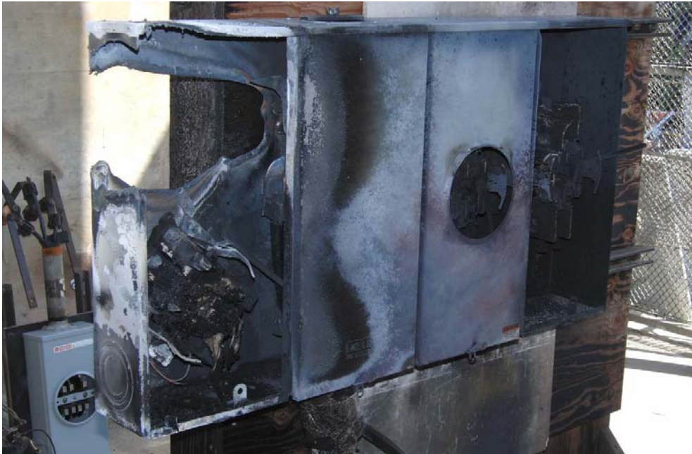
Multi-Meter Sockets Post-Test
