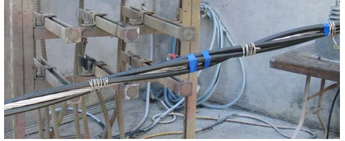
Fig. 13 Overhead quadraplex cable
