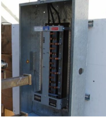
Fig. 11 Small panelboard, 50A-100A
