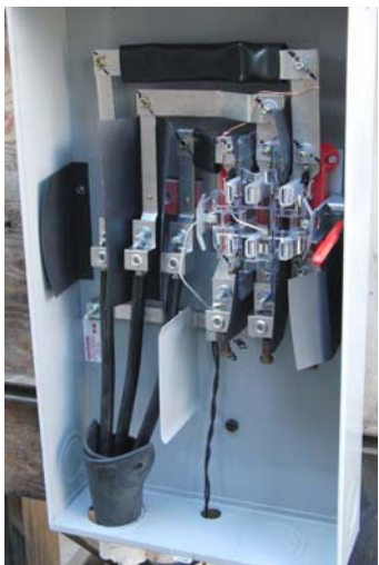
Fig. 16 320-A meter socket with bypass switch
