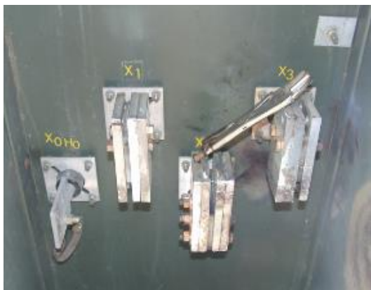
Fig. 7 Padmounted transformer secondary compartment
