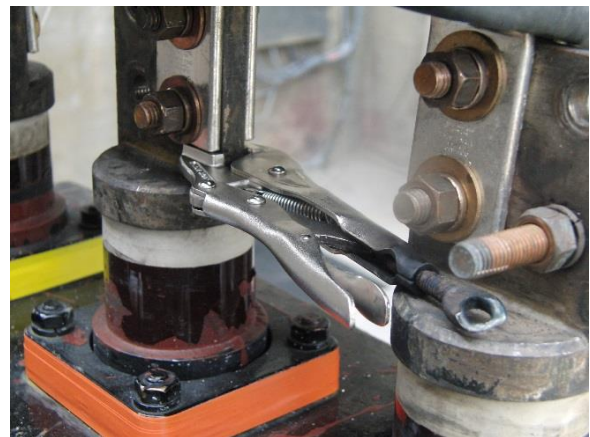
Fig. 22 NP Tool placed phase to phase- 2.65 cycles
