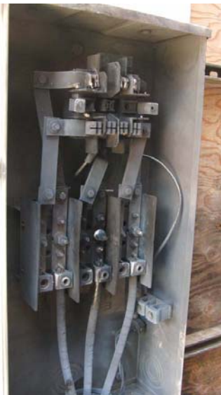
Test Specimen from Fig 15 Post-Test
