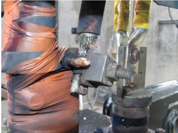
Fig. 23 Loose termination phase to phase- 1.09 cycles
