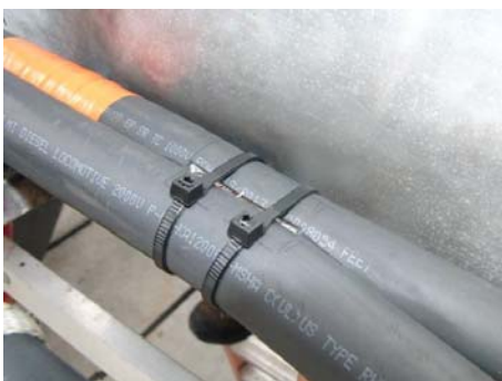
Fig. 25 Phase to phase in cable tray- 1.54 cycles
