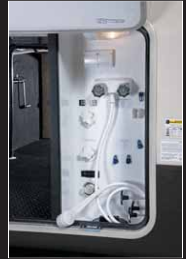
Water management system
