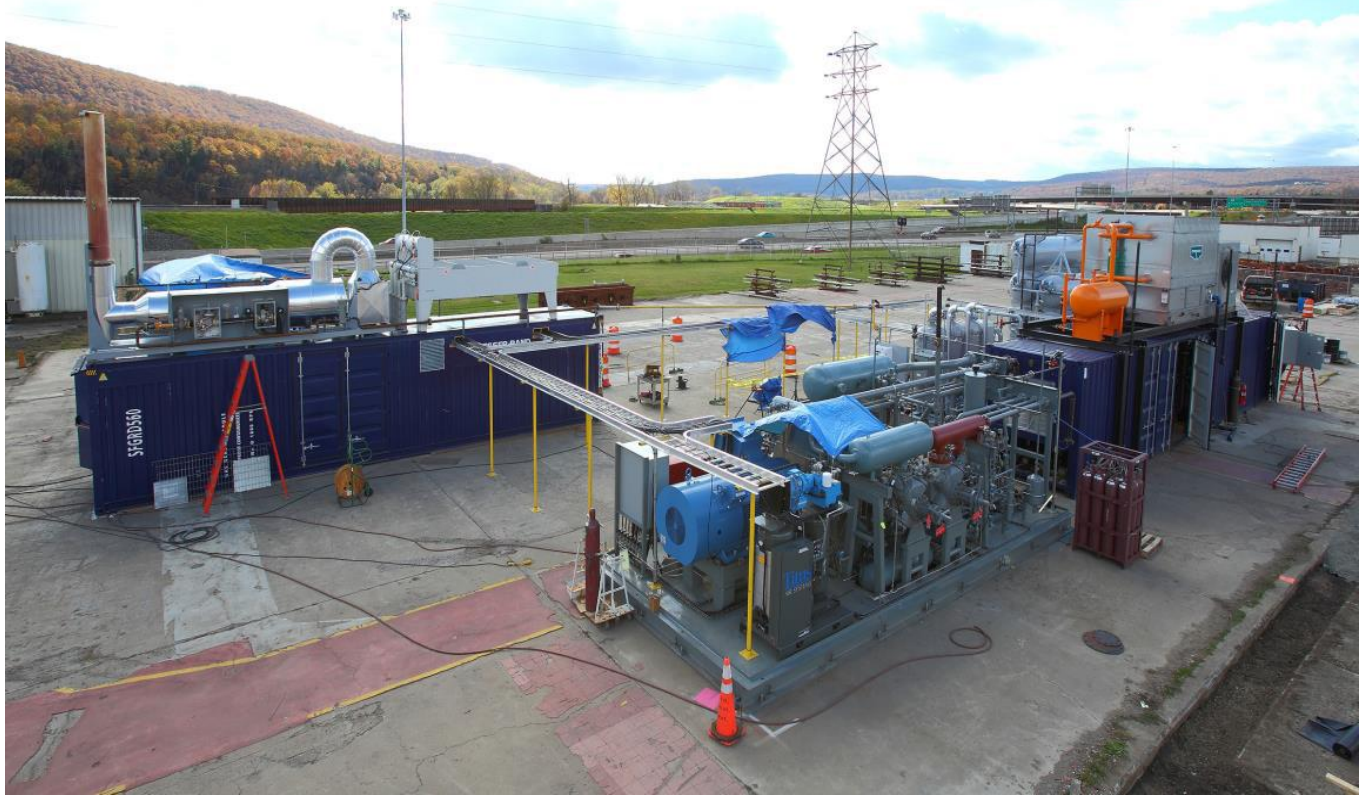
Fully Installed Lngo Plant
