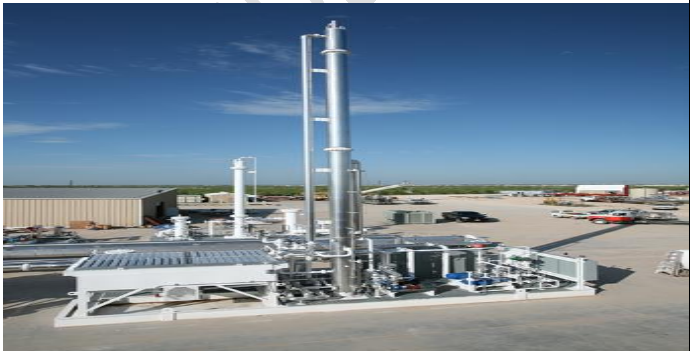
Fully Installed "Amine" Gas Treatment Plant
