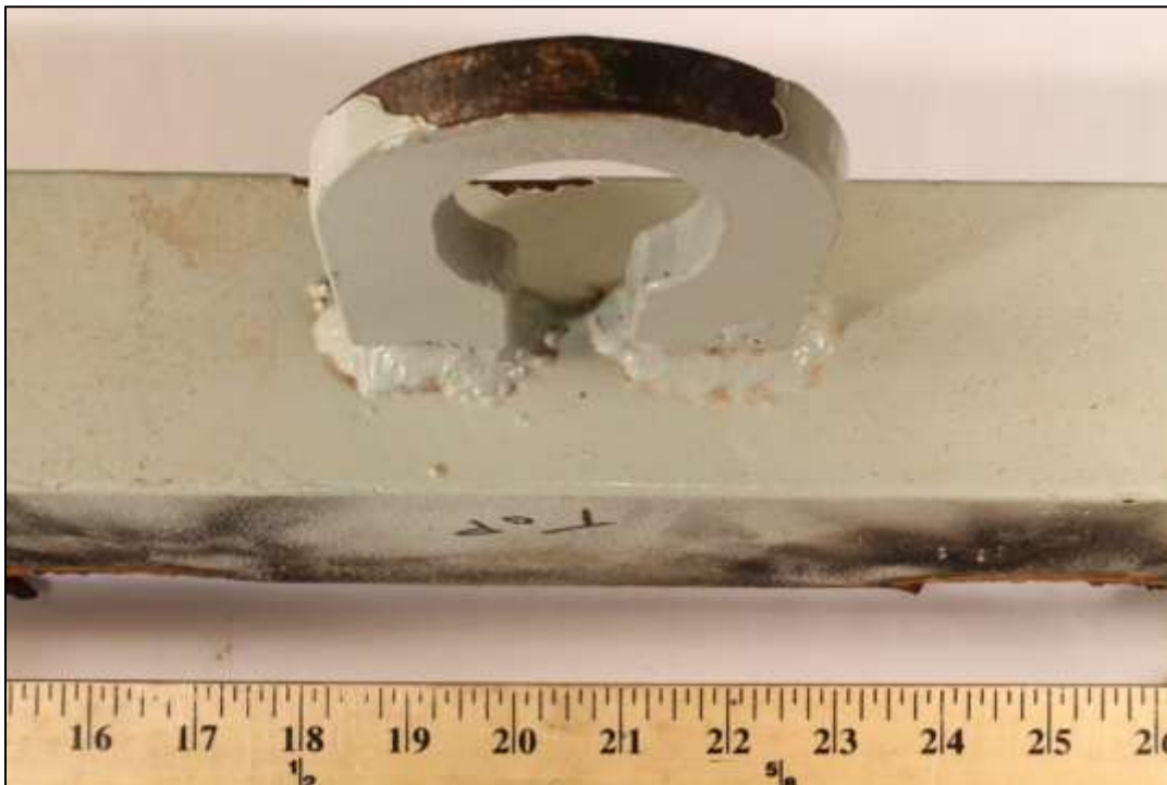
Photo 6 – MATCO photo of removed intact lug showing fillet weld connection to the stiffening angle. This lug was near the bottom of the door and was not being used when the accident occurred. Arrow points in the direction of the top of the door.
