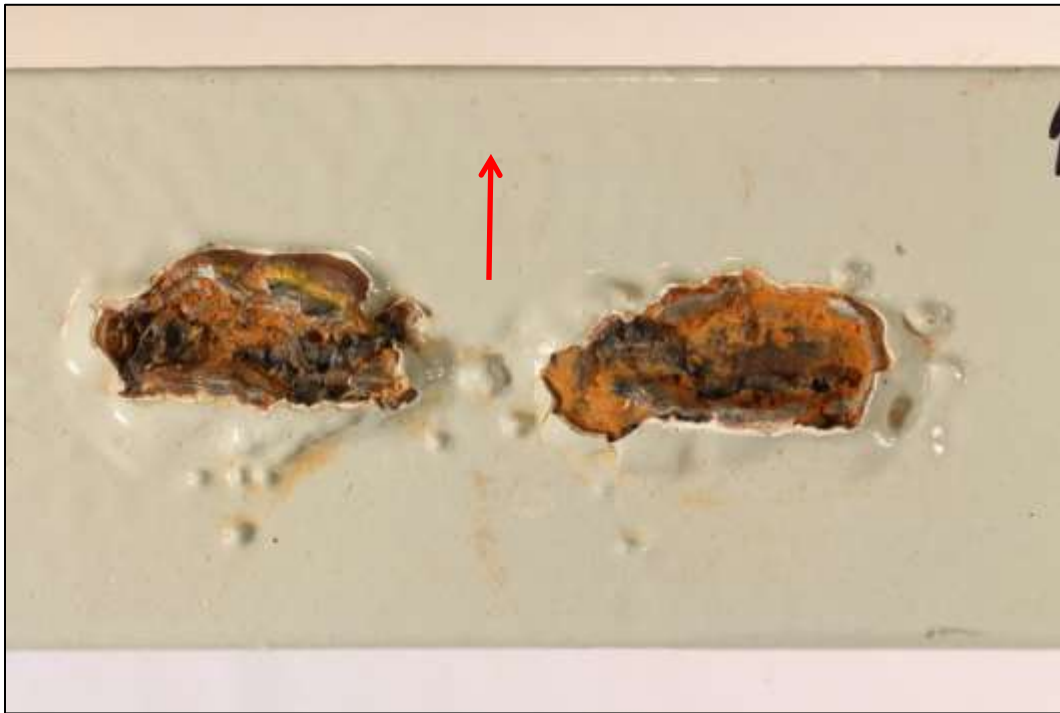
Photo 5 – MATCO photo of fractured welds on tank door stiffening angle. Arrow points to the top of the door.
