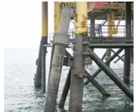
Riser bearing bonding
