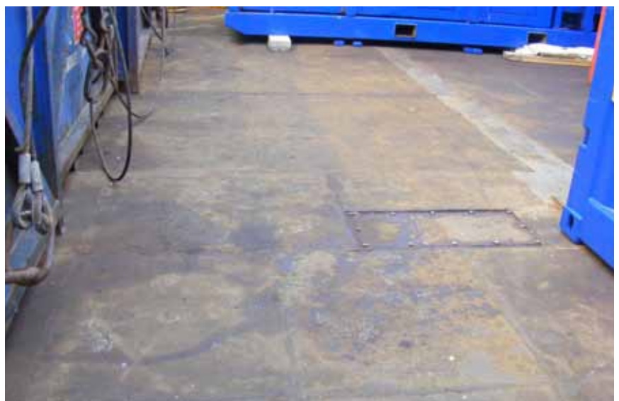
8 years later, Belzona plate bonding solution in excellent condition
