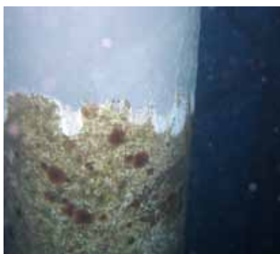
Corroded platform leg
