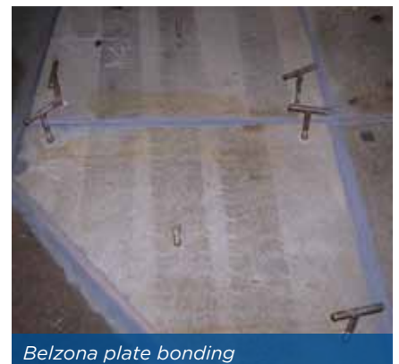
Corroded deck, North Sea platform
