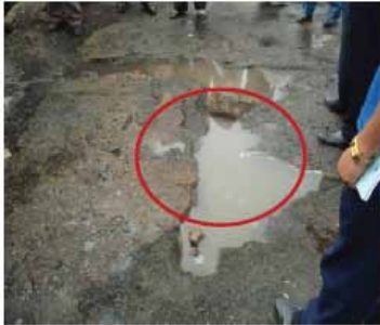
Bad cracks and holes on road
