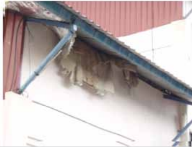
Leaking roof at community hall
