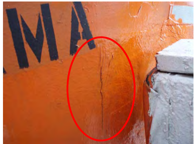
Damage of shell
