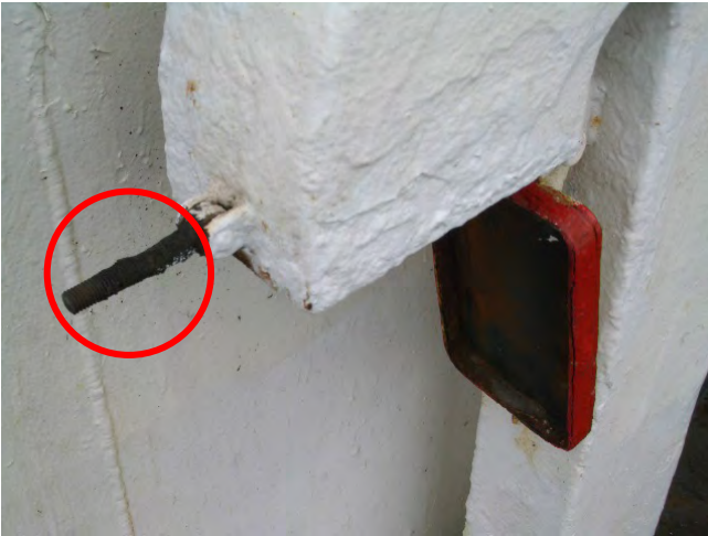
Missing butterfly nut of gooseneck ventilator
