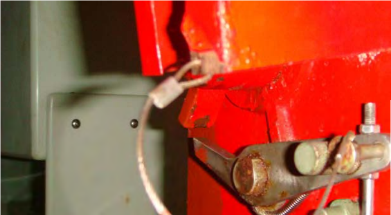
Incorrect position of the lever
