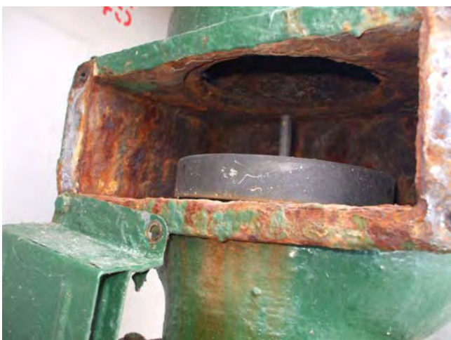
Wastage of inside of air pipe head
