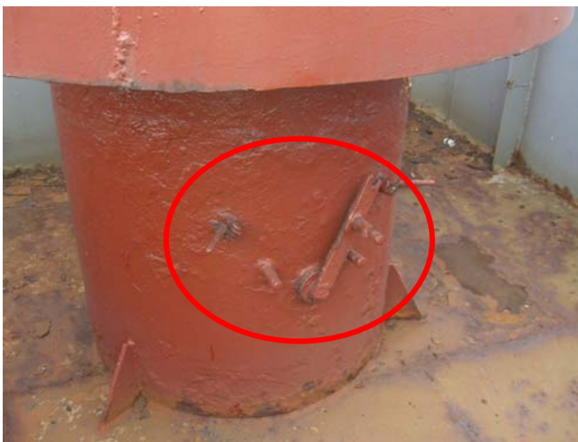
No marking of “Close-Open”
