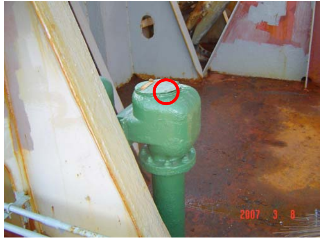
Missing bolt of air pipe head
