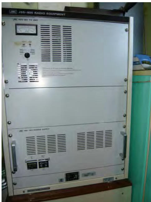
Switch Panel for MF/HF radio
