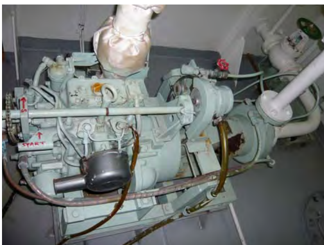
Emergency fire pump
