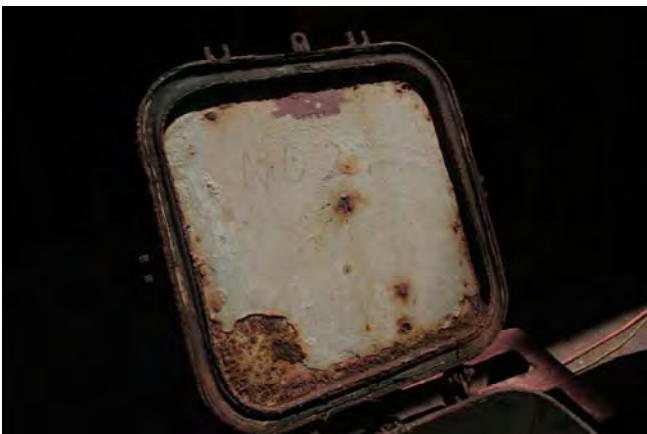
Deteriorated rubber packing
