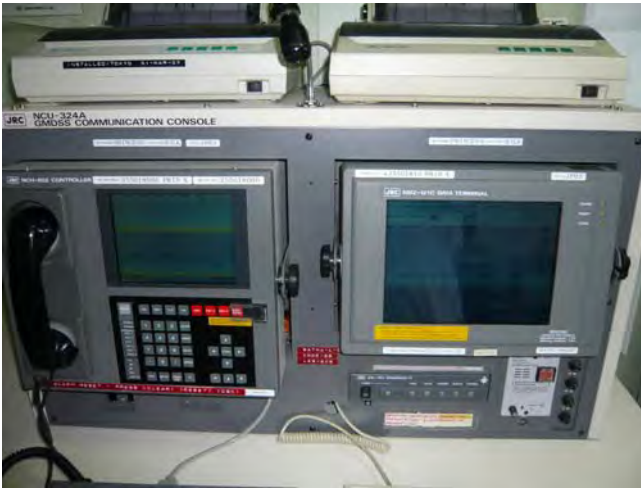
GMDSS communication console
