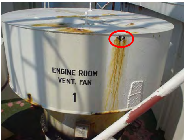
Holes of the casing of ventilator
