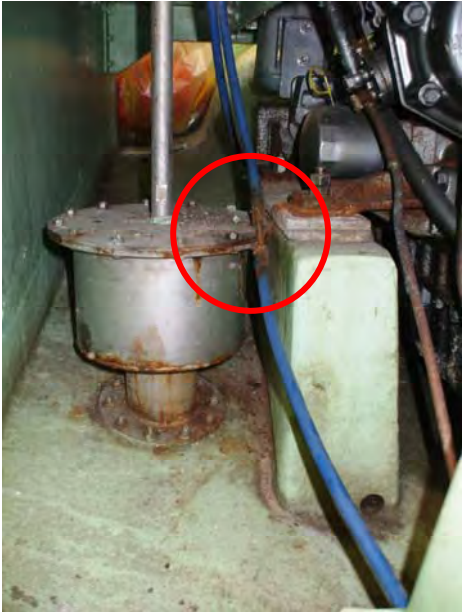
Defective release cable
