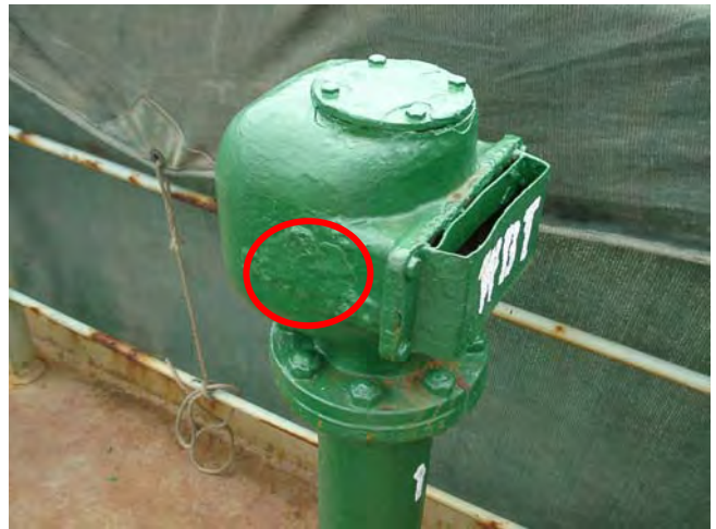
Temporary repaired by patty → Not acceptable!
