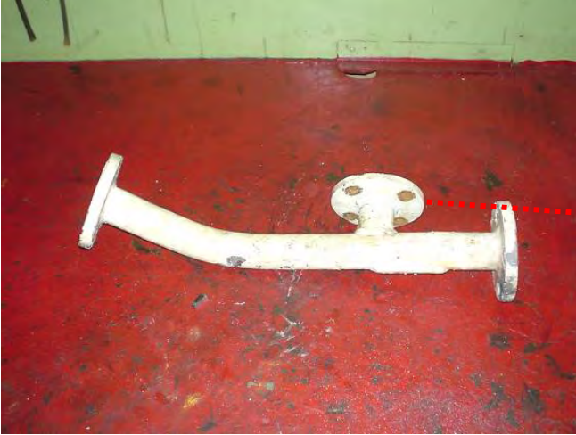
Flange connection to by-pass line
