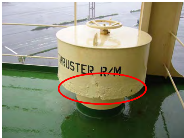
Wastage of the casing of ventilator
