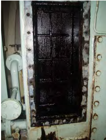
Oily inside of oil water separator
