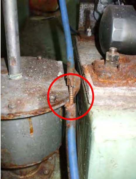
Defective release cable
