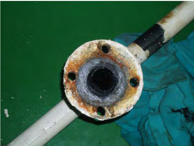
Oily inside of discharge pipe
