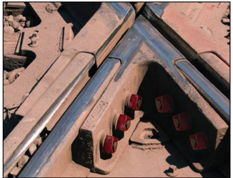
FIGURE 5: The Huck 360® lock bolt system installed on BNSF Railway's Opal Diamond at Temple, Texas.
