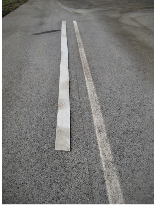
Figure 12: Thermoplastic Repositioned After Failure
