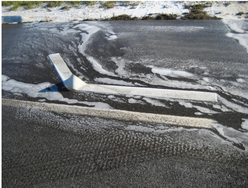
Figure 11: Catastrophic Failure of Thermoplastic
