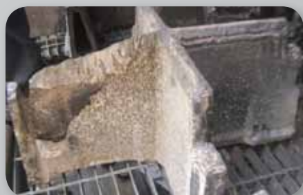
Burner tip: after wear
