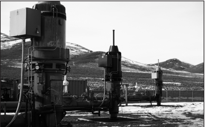
Geothermal production wells, at McGinness Hills Field, Lander County (Lowell Price photo).
