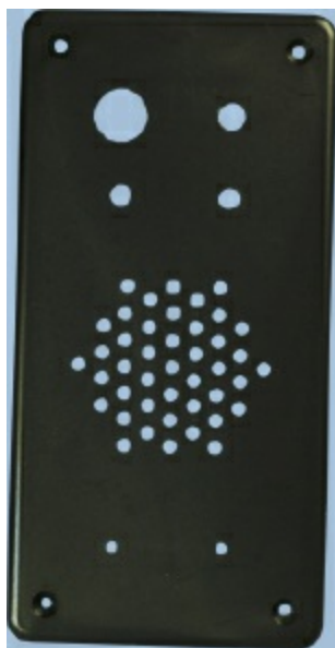
Figure 3-108. The exterior of the panel after drilling. A small handheld cordless drill can create a neat result if the holes were marked carefully.
