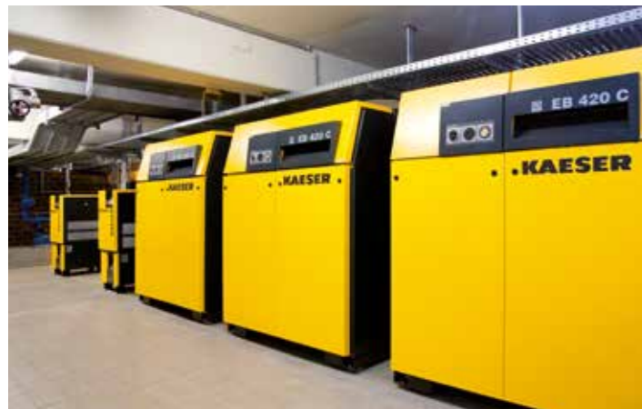
In the Jägersburg waterworks of the Wasserbeschaffungsverband Riedgruppe Ost, KAESER rotary blowers are coordinated and regulated by the central control system, ensuring the safe, efficient backwashing of the sand filters
