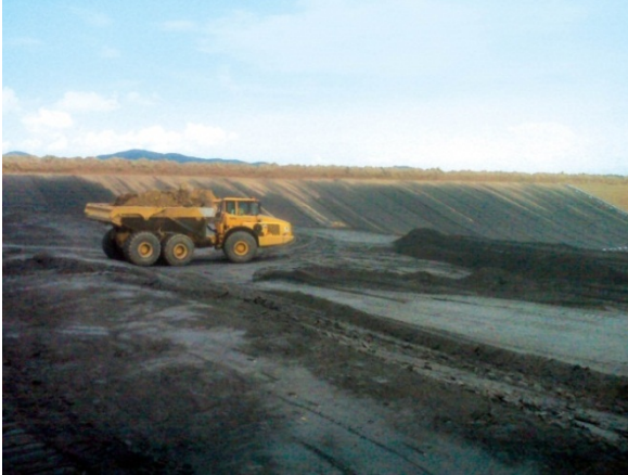
Figure 17. Large Un-vegetated Surfaces
