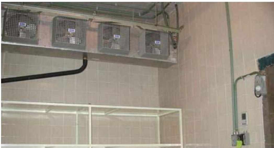
Figure 33. Cooling room for mangoes.
