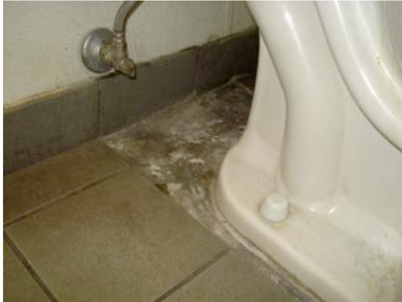
Figure 32 Dirt behind a Toilet
