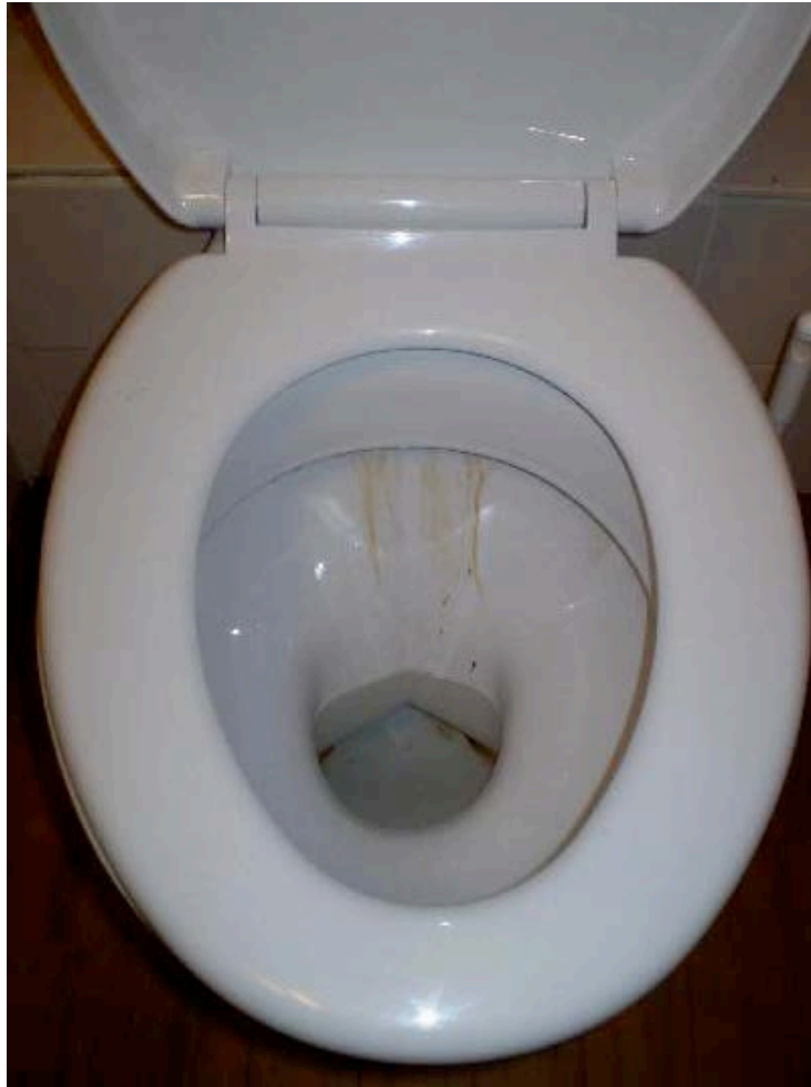
Figure 45 Dirty toilet bowl and hole at bottom
