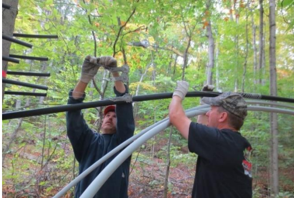
Figure 37 - Installation of a mainline Mainline installation at Shelburne Farms. A wire mesh tension grip is being used to anchor the mainline to the support wire. (Image source Shelburne Farms, n.d.)
