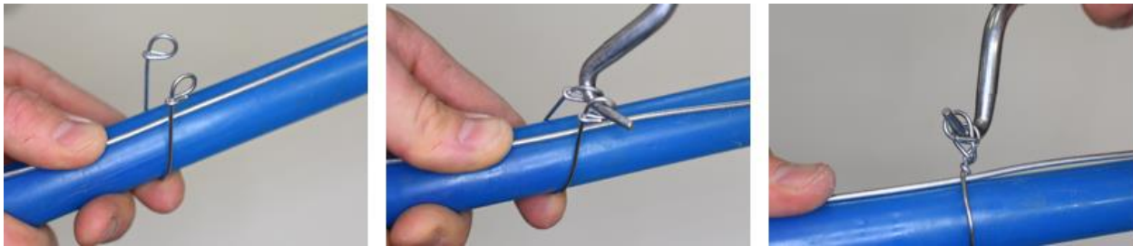
Figure 38 - Connecting support wire to mainline The mainline is attached to the support wire using wire ties. The wire tie is attached using a manual wire twister. (Image source Isselhardt, 2019)
