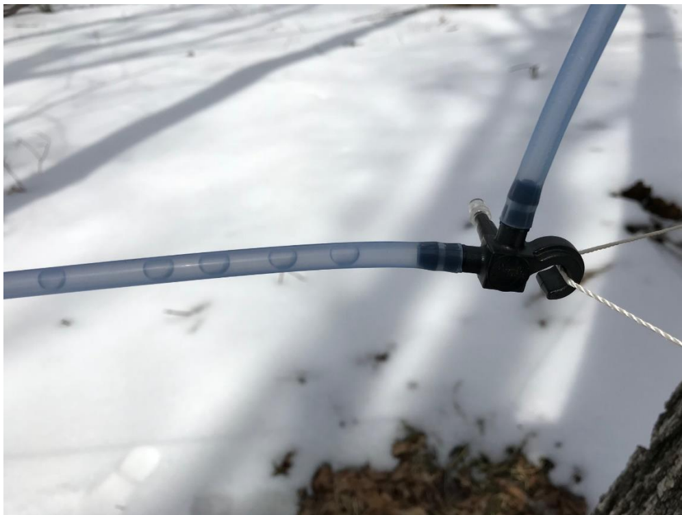
Figure 16. Vacuum tubing leaking at a connector.
