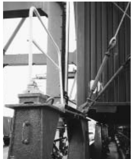
Good example of a safety barrier but note the bridging platform that slots into the outboard platform is not shown.
