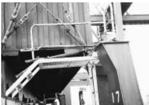
AFTER - The construction of a lashing platform and access ladder, to allow safe access. This particular platform is collapsible to allow the removal of hatch covers.
