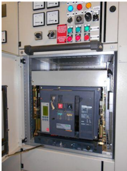
Switch nr. 901 (picture taken from Costa Favolosa)
