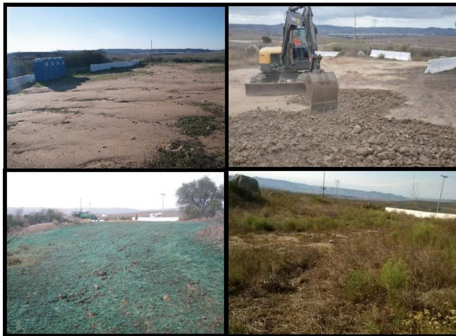
Figure 5. Area A: Before Treatment, During Surface Scarifying/Roughing, Hydro Seeded, and After Treatment; Looking South.
