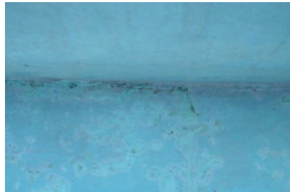
Fig 2 Sealant at keel joint
