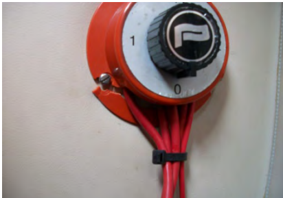
Fig 36 Broken isolator switch
