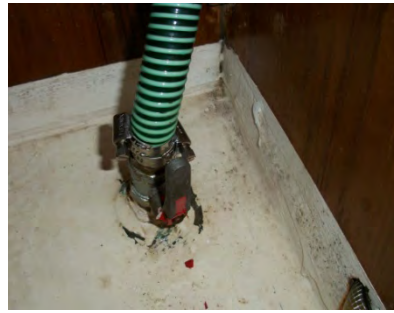
Fig 26 Galley sinks drain
