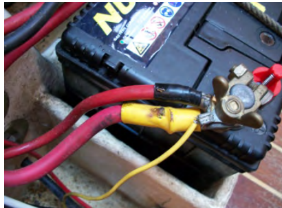
Fig 37 Cranking battery hot terminal
