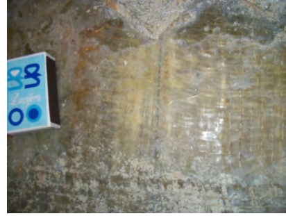
Fig 6 Lighter area is suspected damaged laminate
