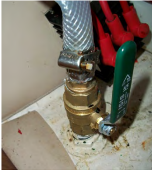
Fig 25 Toilet water intake
