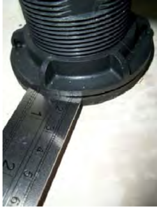
Fig 27 Log thru hull not tight to hull inside yacht.
