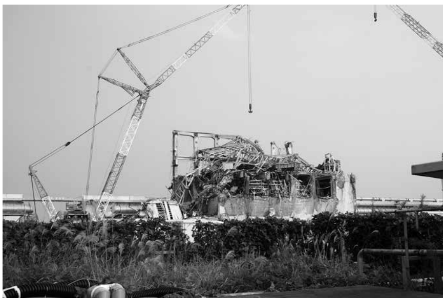
Figure 5.1. The damaged Fukushima Daiichi Reactor Unit 3. Credit: Giovanni Verlini and IEAE, www.flickr.com .
