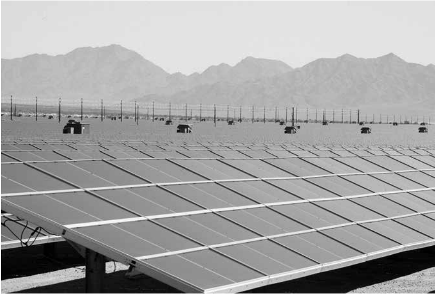
Figure 5.3. The world's largest solar farm located in California: First Solar Desert Sunlight Solar Farm. Credit: US Department of the Interior and www.flickr.com .
