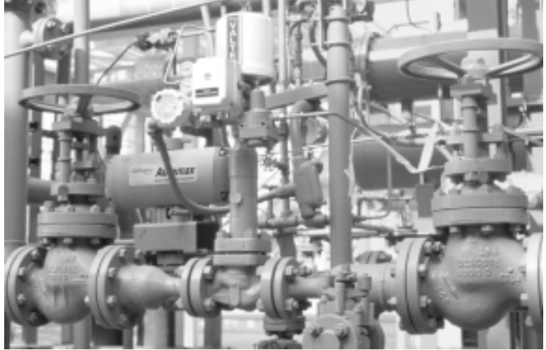
This 2-inch Guardian II operates in a chemical plant.
