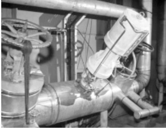
A 4-inch Mark One with side-mounted handwheel operates in a boiler feedwater system at a pulp plant.
