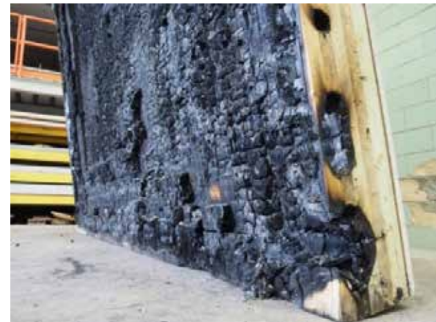
Wall assembly after testing showing the depth of charring on the exposed side. NRC (2014) Fire Endurance of Cross-Laminated Timber Floor and Wall Assemblies for Tall Wood Buildings.
