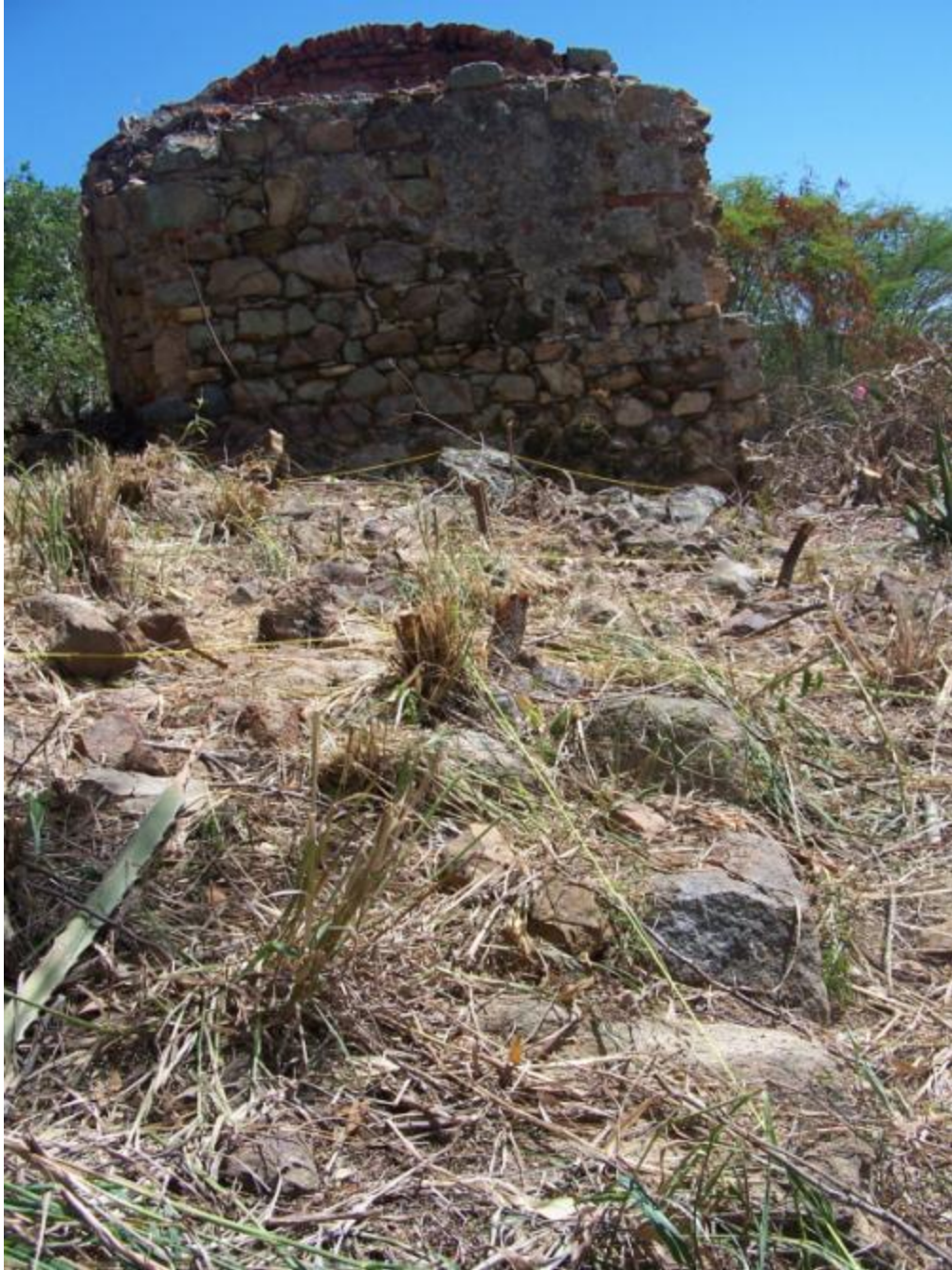
Figure 5-8. Foundation B, facing southwest towards the cistern. Photo taken in 2008 by the author.
