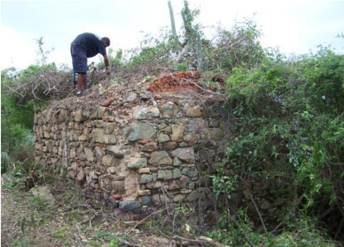
Figure 5-3. Clearing of brush from the cistern. Photo taken by the author in 2008.
