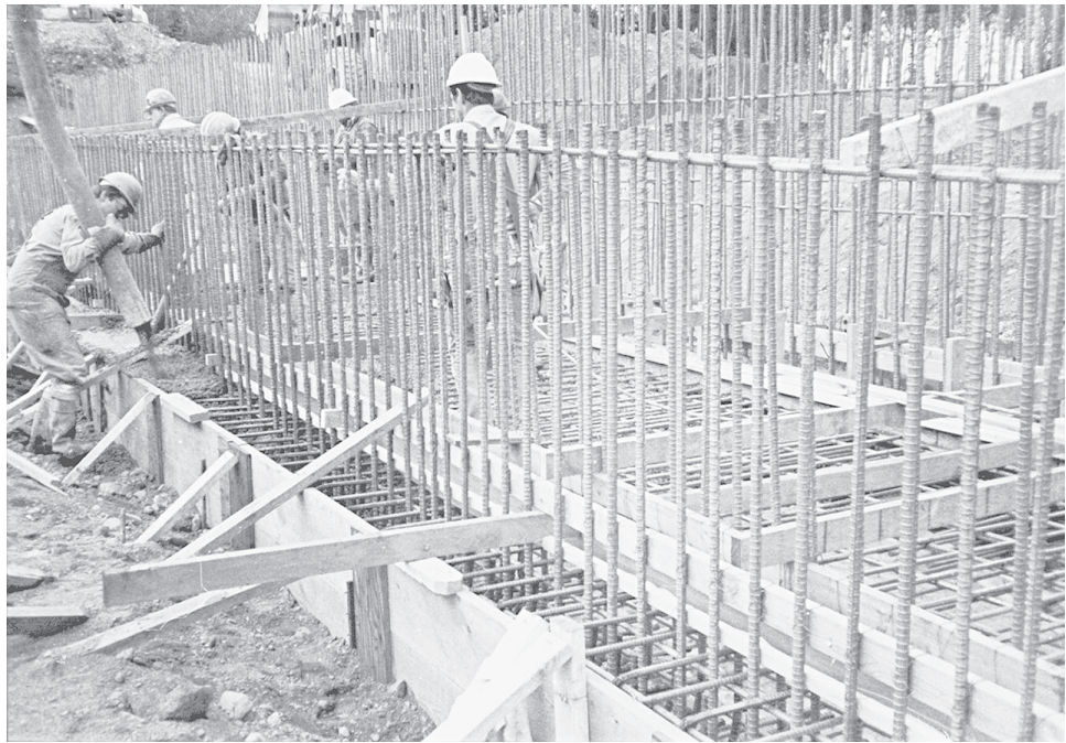
FIGURE 1-5 Concrete construction in progress. Note formwork, reinforcing bars, and pumping of concrete.
