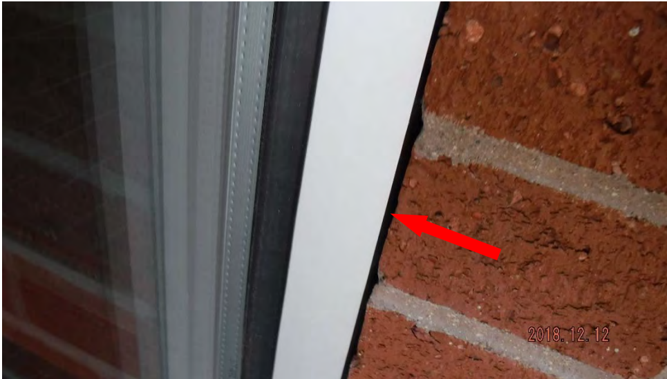
6a. Gap between masonry and window/door frame (see #6 on elevation photo for location).
