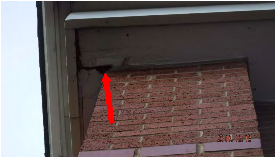
4a. Disrepair of soffit and chipping/flaking paint (see #4 on elevation photo for typical location).
