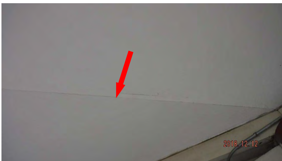
2b. Cracks in soffit ceiling (see #2 on elevation photo for typical location).
