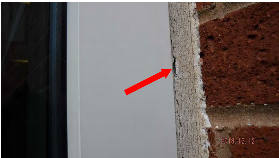
5b. Cracking/shrunk sealant joint (see #5 on elevation photo for typical location).
