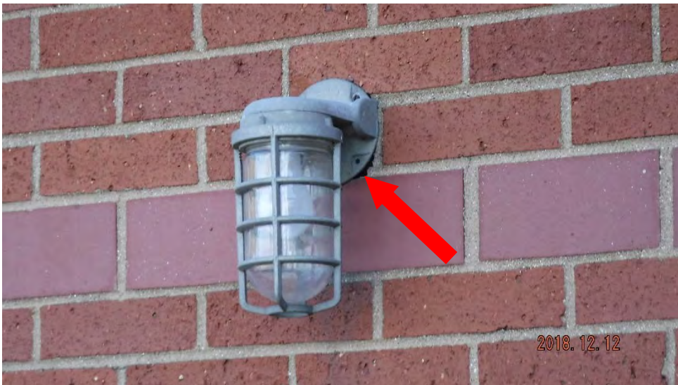
1b. Open joint between penetration and veneer (see #1 on elevation photo for location).
