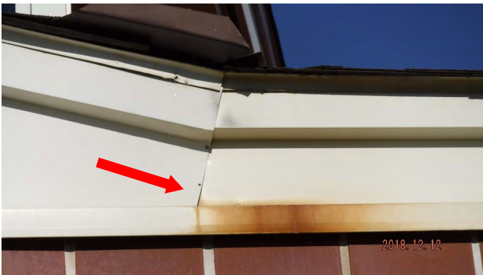
4a. Loose fascia metal and corrosion on cap/drip metal (see #4 on elevation photo for location).
