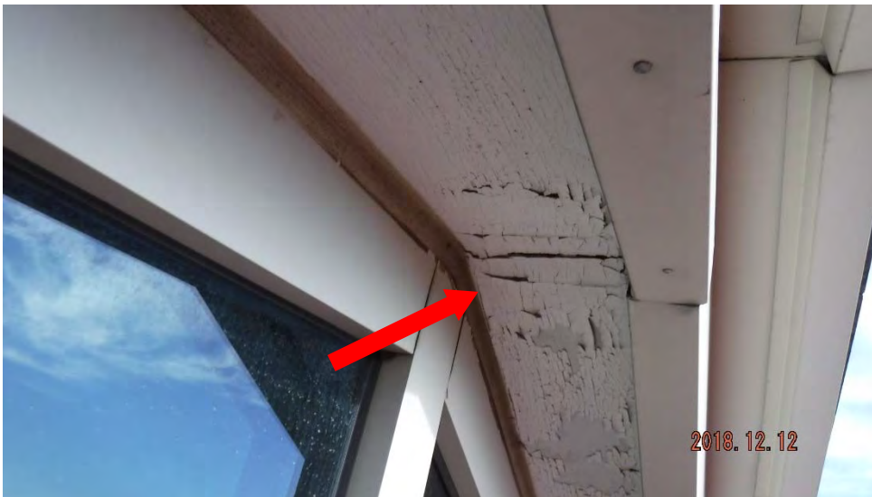
1b. Chipping/flaking paint (see #1 on elevation photo for typical location).
