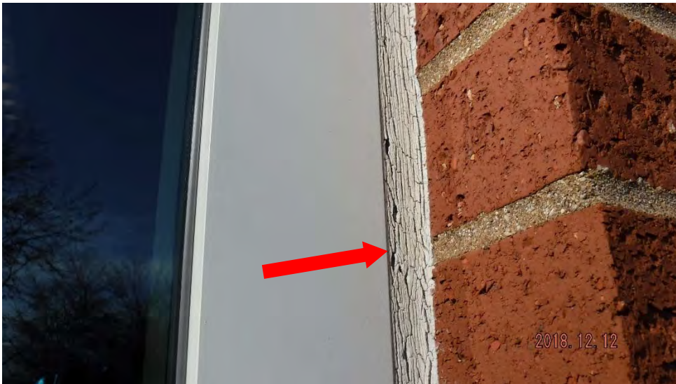
5d. Cracking/shrunk sealant joint (see #5 on elevation photo for typical location).
