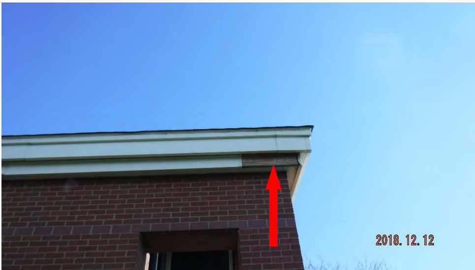
5a. Overview of area where fascia metal is missing (see #5 on elevation photo for location).
