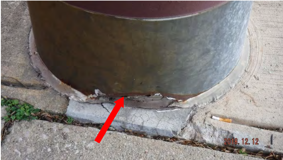
3c. Corrosion at base of steel column (see #3 on elevation photo for location).
