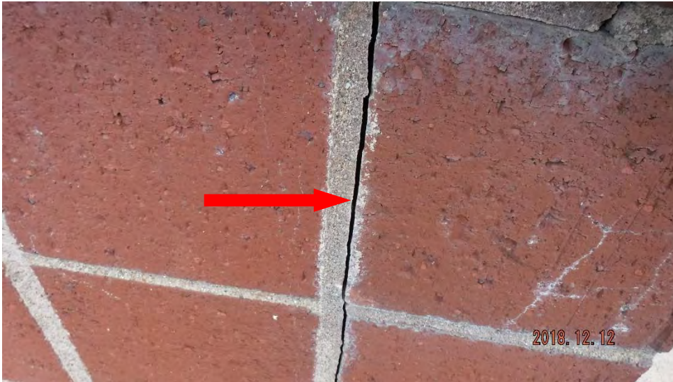
1c. Cracked/shrunk mortar joint (see #1 on elevation photo for typical location).
