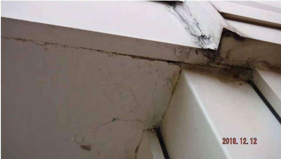
2c. Deterioration of soffit ceiling and chipping/flaking paint (see #2 on elevation photo for typical location).
