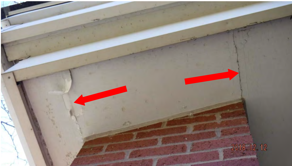
4d. Cracked joint, delaminating tape, and chipping/flaking paint (see #4 on elevation photo for typical location).
