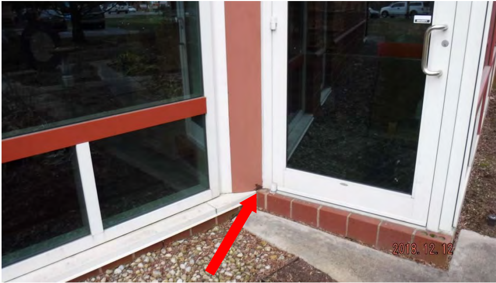
6a. Overview of steel column. See area of corrosion at arrow (see #6 on elevation photo for location).
