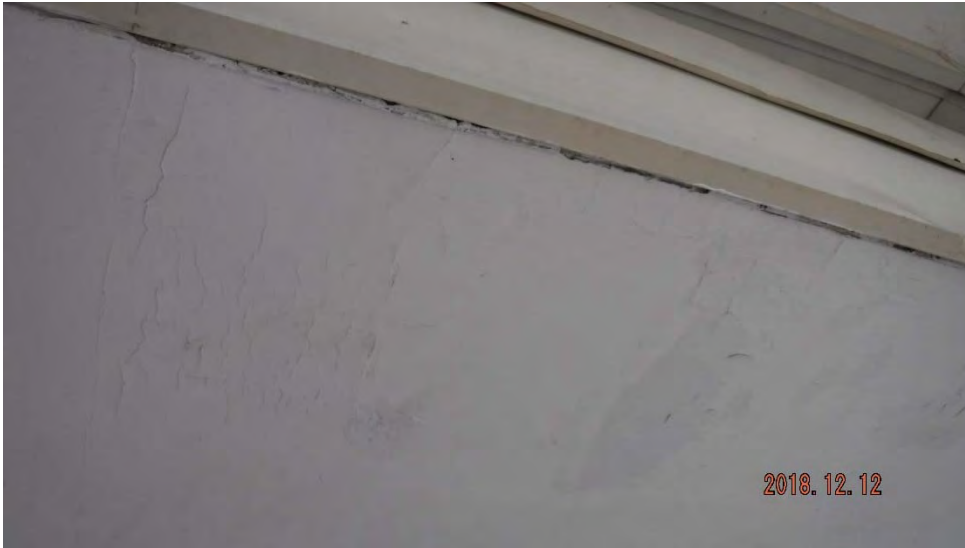
2g. Deterioration of soffit ceiling and chipping/flaking paint (see #2 on elevation photo for typical location).
