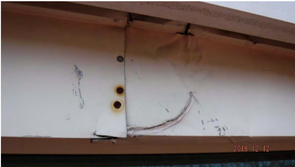
1b. Damaged fascia metal (see #1 on plan view for location).
