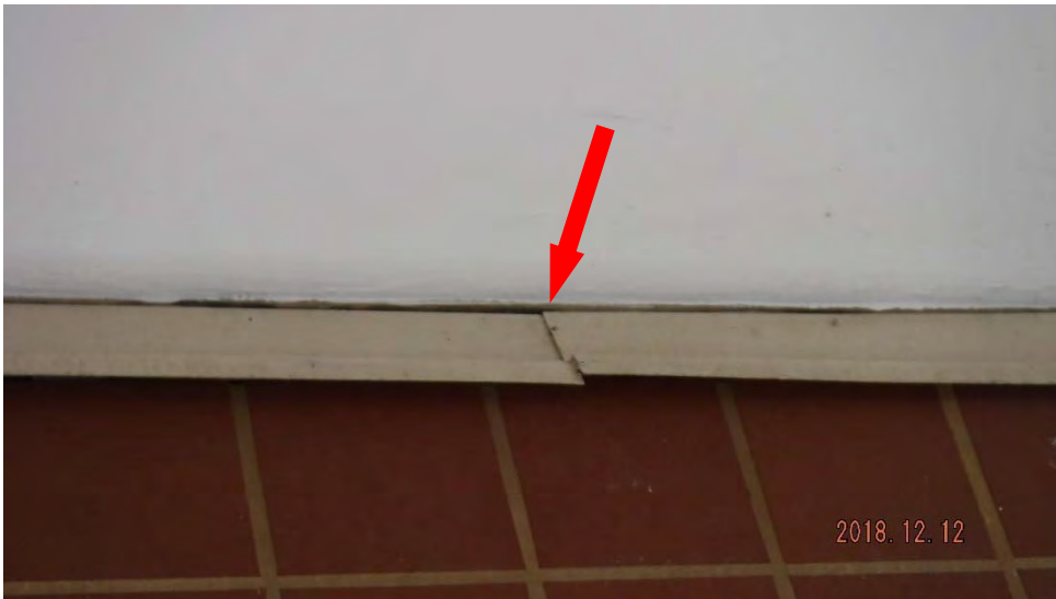
2h. Loose metal flashing (see #2 on elevation photo for typical location).
