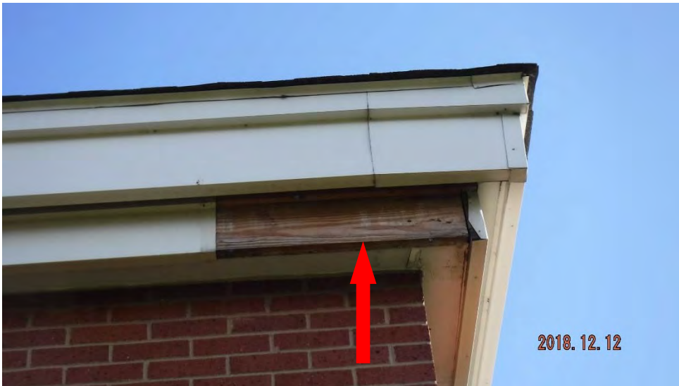
5b. Exposed wood member where fascia metal is missing (see #5 on elevation photo for location).
