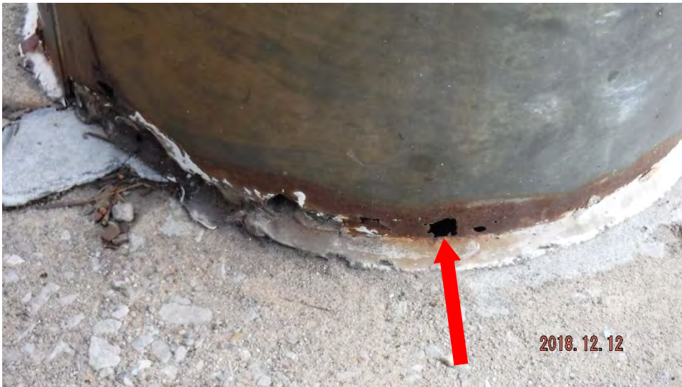
3d. Severe corrosion at base of steel column (see #3 on elevation photo for location).
