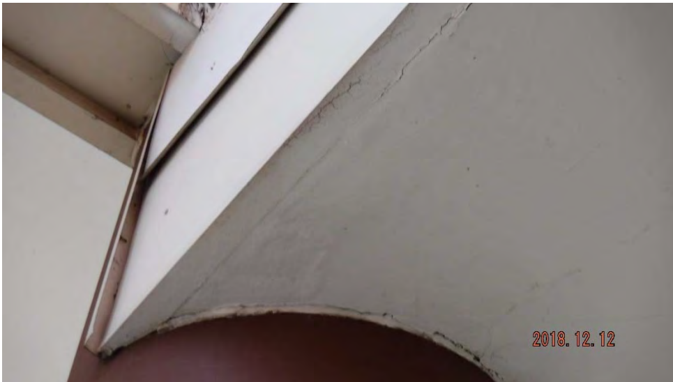
2d. Deterioration of soffit ceiling and chipping/flaking paint (see #2 on elevation photo for typical location).
