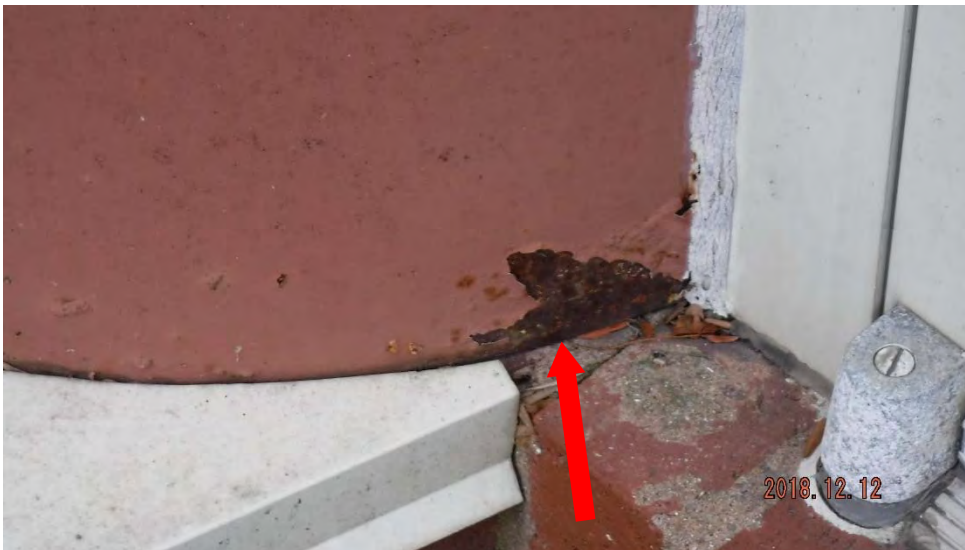
6b. Corrosion at base of steel column (see #6 on elevation photo for location).
