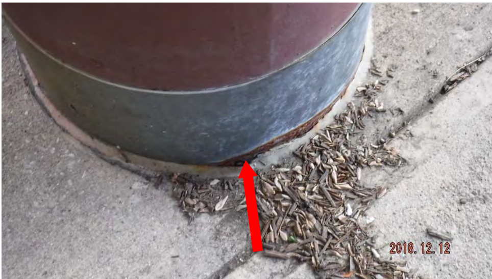
3b. Corrosion at base of steel column (see #3 on elevation photo for location).
