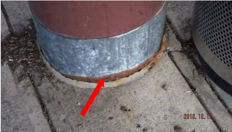
3a. Corrosion at base of steel column (see #3 on elevation photo for location).
