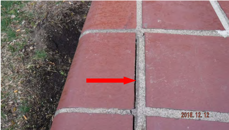
1e. Cracked/shrunk mortar joint(s) (see #1 on elevation photo for typical location).
