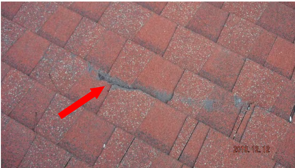
3b. Damaged shingles (see #3 on plan view for location).
