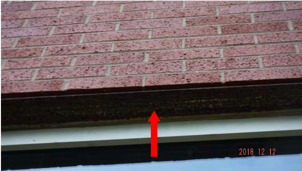
3b. Corrosion on window lintel (see #3 on elevation photo for location).
