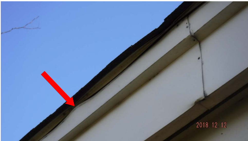
3b. Drip edge metal not lapping over fascia metal as required (see #3 on elevation photo for location).
