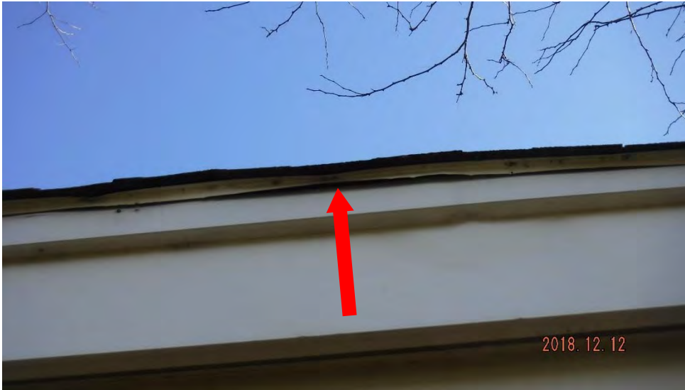
3a. Damaged or distorted drip edge metal (see #3 on elevation photo for location).
