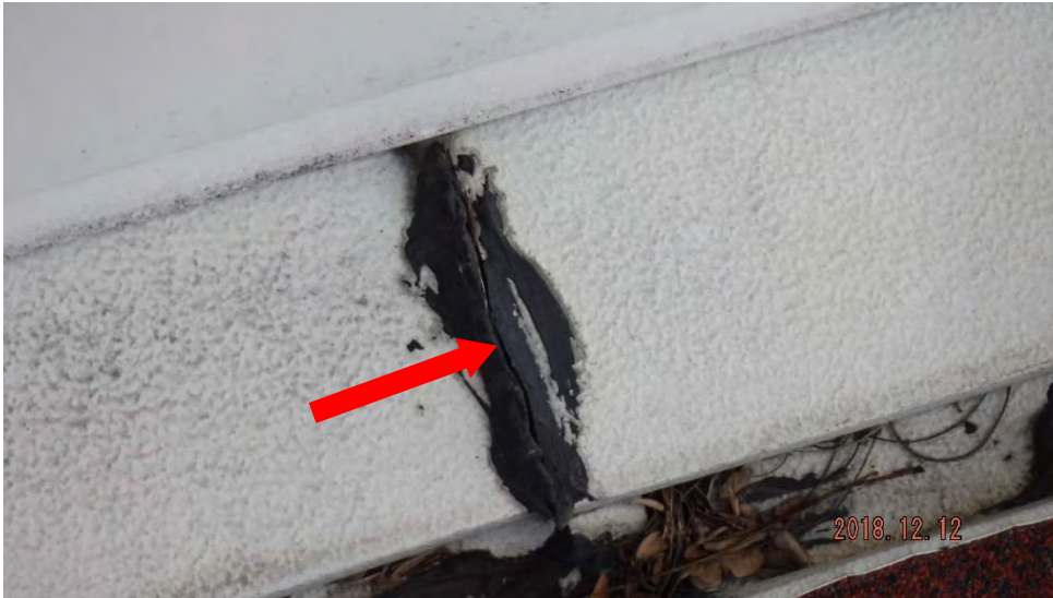
2d. Cracking of the sealant at the vent joint (see #2 on plan view for typical location).
