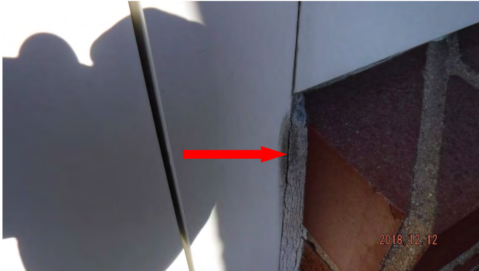
2b. Cracked/shrunk sealant joint (see #2 on elevation photo for location).
