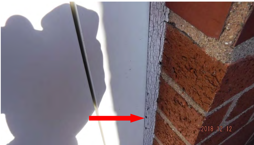
2a. Cracked/shrunk sealant joint (see #2 on elevation photo for location).
