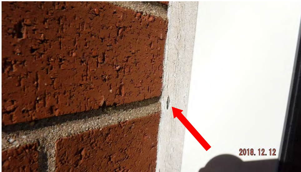
1a. Cracking/shrunk sealant joint. Exposed backer rod visible (see #1 on elevation photo for typical location).
