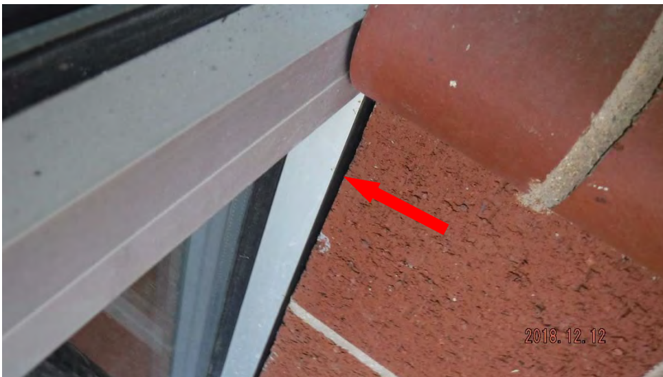
6b. Gap between masonry and window/door frame (see #6 on elevation photo for location).
