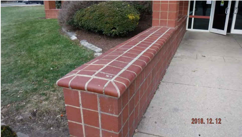
1a. Freestanding wall at main entrance (see #1 on elevation photo for typical location).
