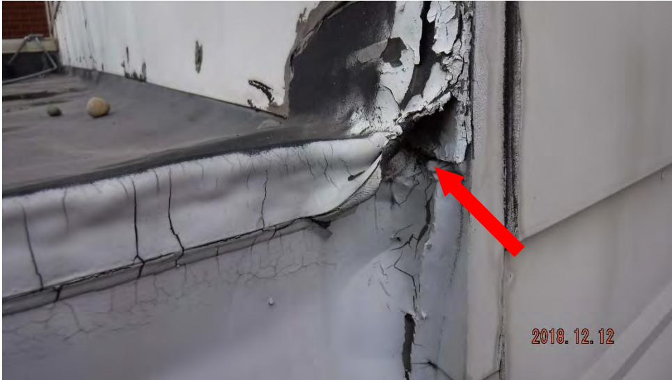
4a. Open flashing at roof edge to wall (see #4 on plan view for approximate location).
