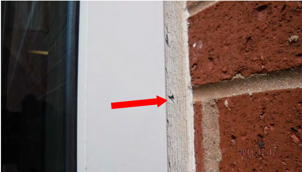
5a. Cracking/shrunk sealant joint (see #5 on elevation photo for typical location).
