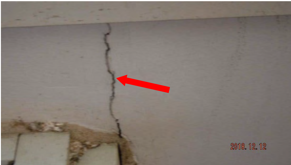
4c. Crack in soffit (see #4 on elevation photo for typical location).
