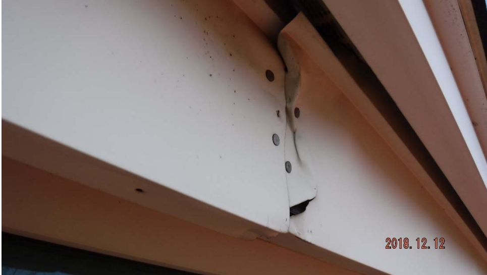
1a. Damaged fascia metal (see #1 on plan view for location).
