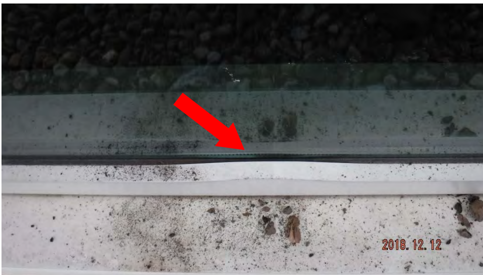
5b. Closer view of damaged pressure plate (see #5 on elevation photo for location).
