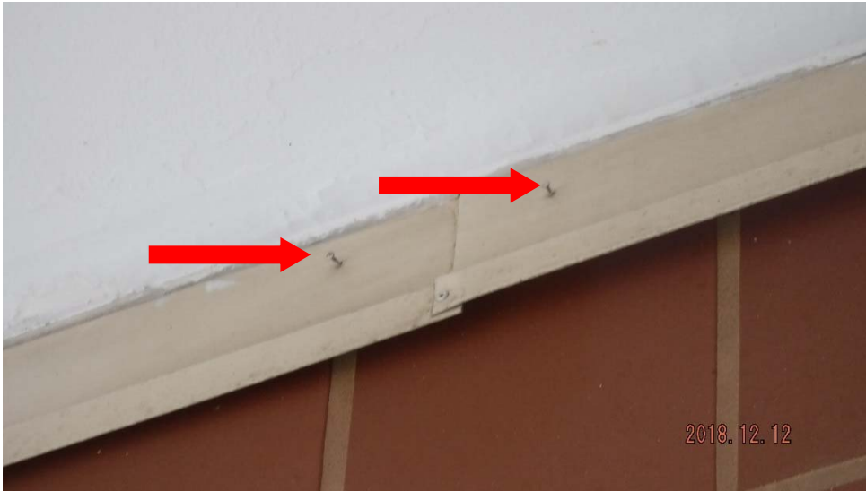
2i. Loose fasteners for metal flashing (see #2 on elevation photo for typical location).
