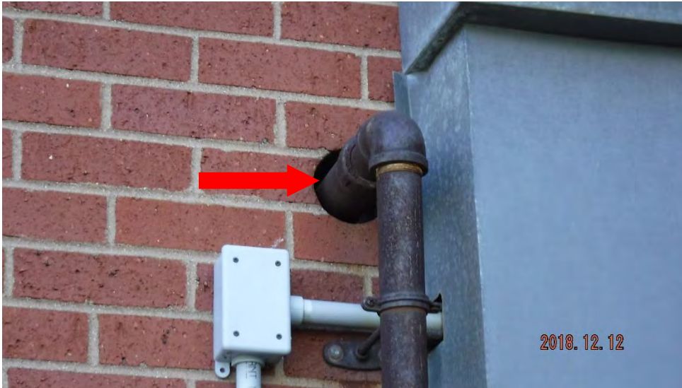
1a. Open joint between penetration and veneer (see #1 on elevation photo for location).
