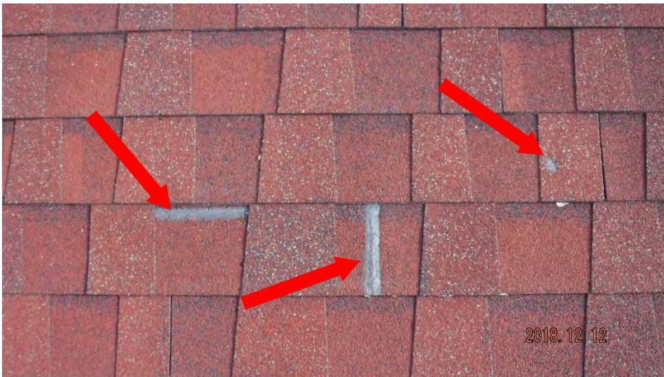
3a. Exposed fabric in deficient shingles (see #3 on plan view for typical locations).
