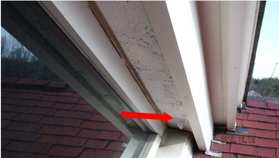
1c. Chipping/flaking paint (see #1 on elevation photo for typical location).
