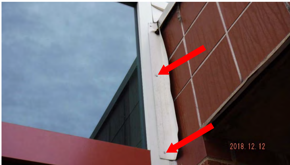
7a. Overall of the metal flashing. See fasteners through fastened into window frame (see #7 on elevation photo for location).
