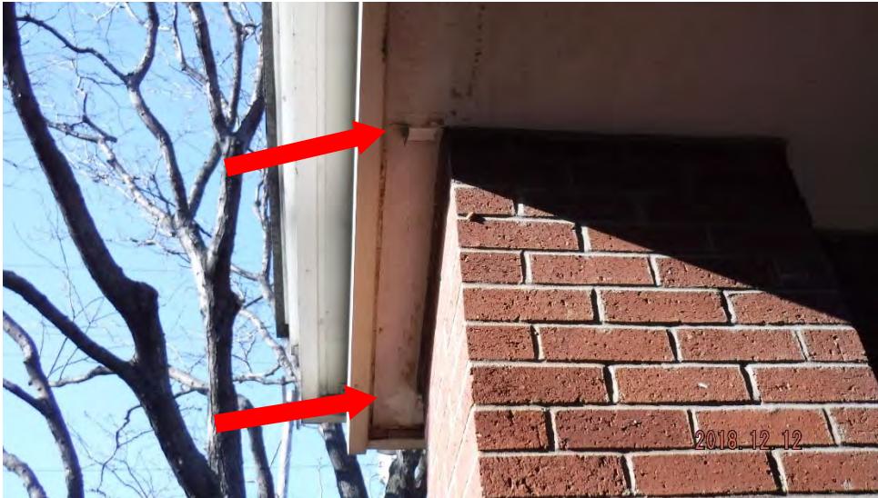
3d. Disrepair of soffit and chipping/flaking paint (see #3 on elevation photo for typical location).
