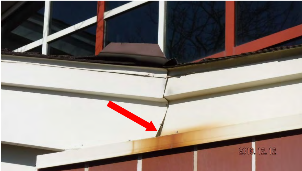
4b. Loose fascia metal and corrosion on cap/drip metal (see #4 on elevation photo for location).
