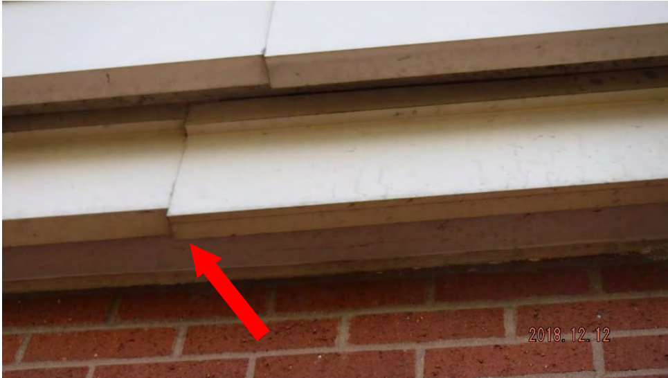
4a. Unsecured/loose fascia metal (see #4 on elevation photo for location).
