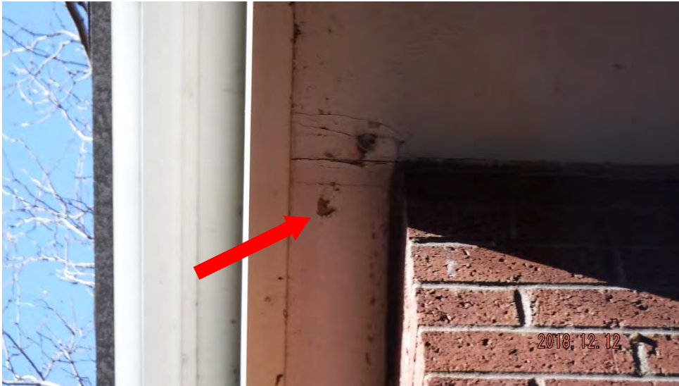
3b. Disrepair of soffit and chipping/flaking paint (see #3 on elevation photo for typical location).
