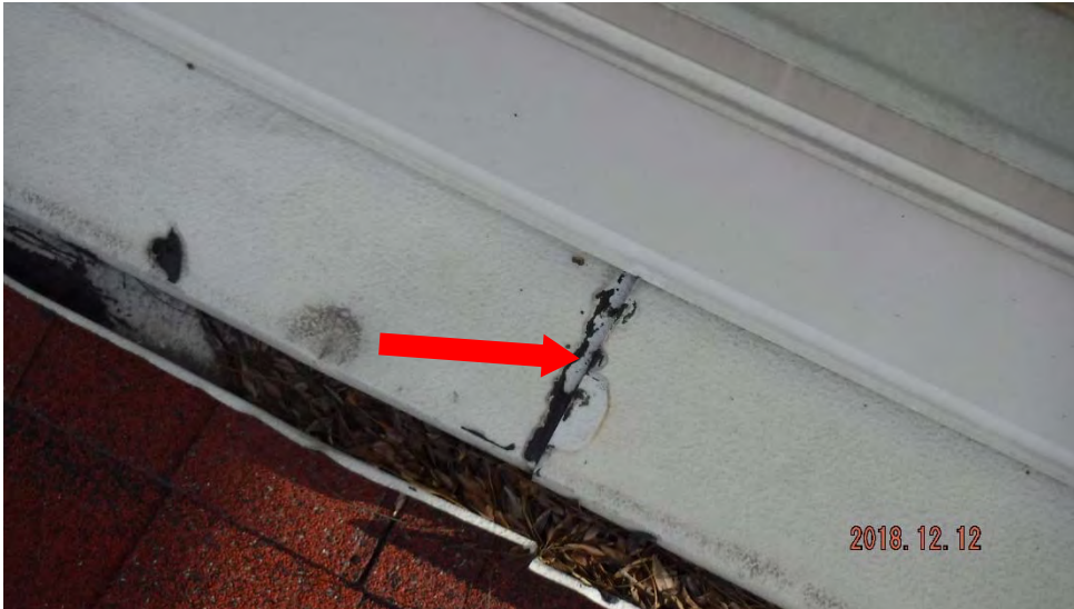
2b. Missing sealant at the vent joint (see #2 on plan view for typical location).
