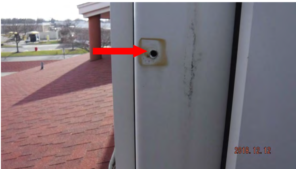
2b. Hole in steel member where item was removed (see #2 on plan view for location).
