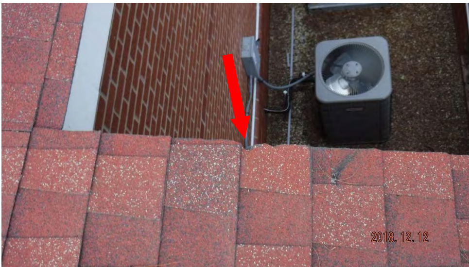
3d. Damaged shingles (see #3 on plan view for location).
