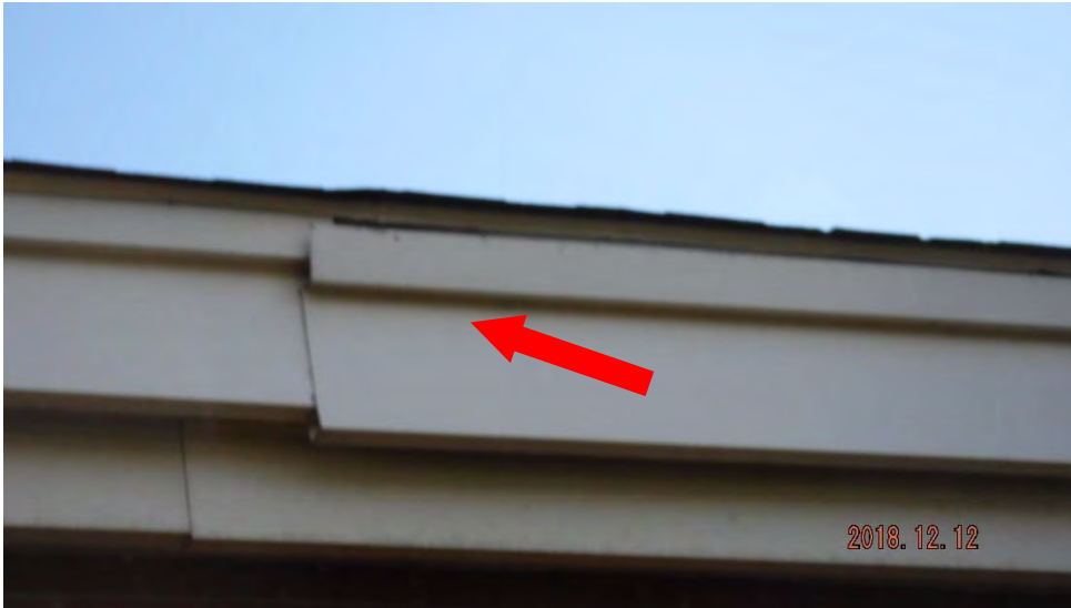
4c. Unsecured/loose fascia metal (see #4 on elevation photo for location).
