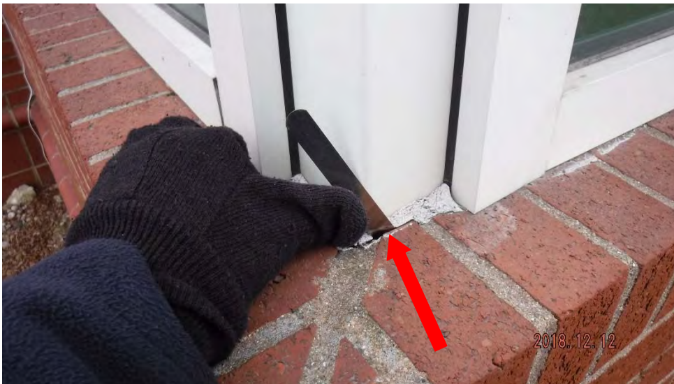
1b. Probe inserted several inches into open space at sealant joint (see #1 on elevation photo for location).
