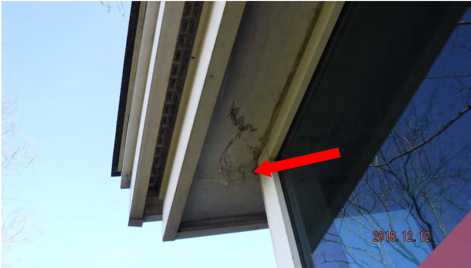
2a. Disrepair of soffit and chipping/flaking paint (see #2 on elevation photo for typical location).
