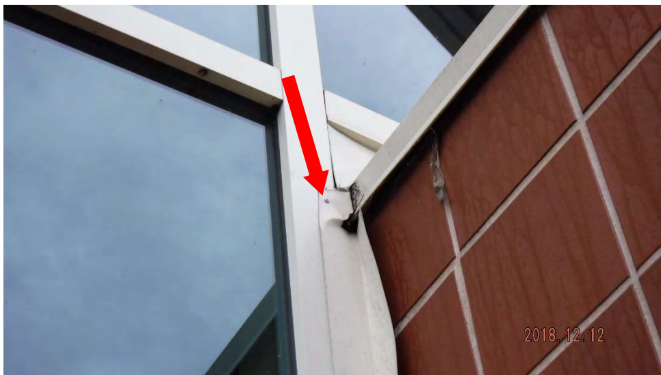
7b. Fastener through fastened into window frame (see #7 on elevation photo for location).
