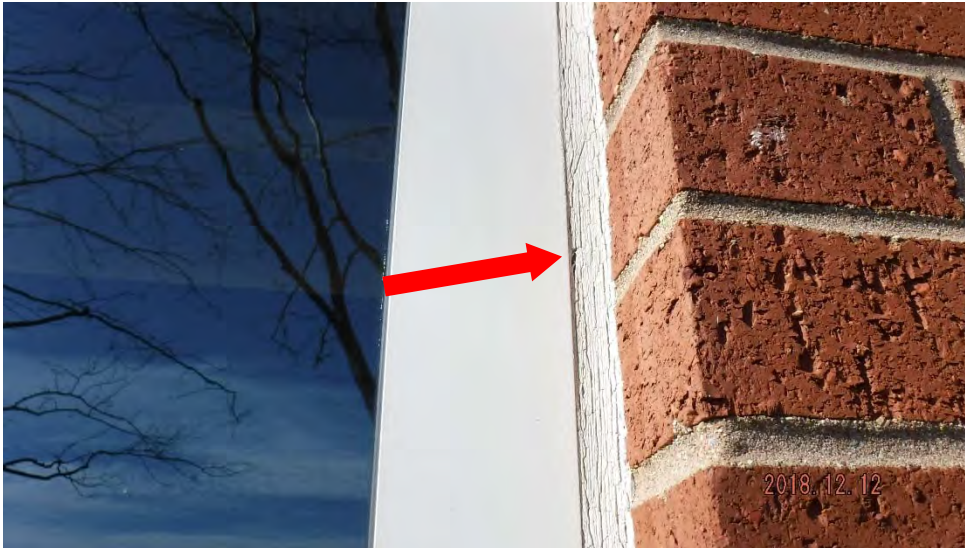
5c. Cracking/shrunk sealant joint (see #5 on elevation photo for typical location).
