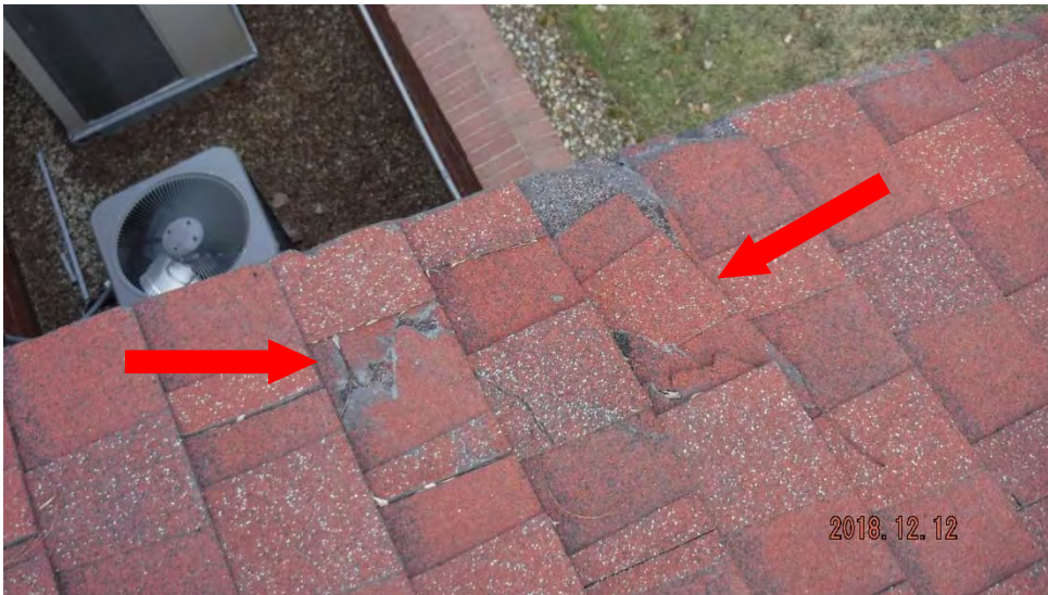
3c. Multiple damaged shingles (see #3 on plan view for location).
