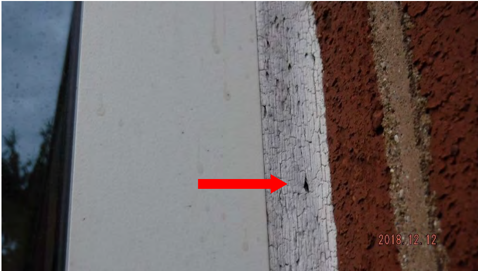
1c. Cracking/shrunk sealant joint (see #1 on elevation photo for typical location).
