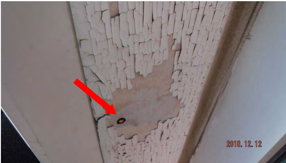
1a. Exposed fastener and chipping/flaking paint (see #1 on elevation photo for typical location).
