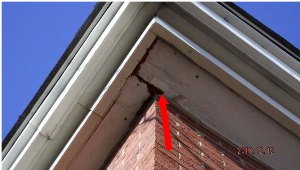
3a. Disrepair of soffit and chipping/flaking paint (see #3 on elevation photo for typical location).
