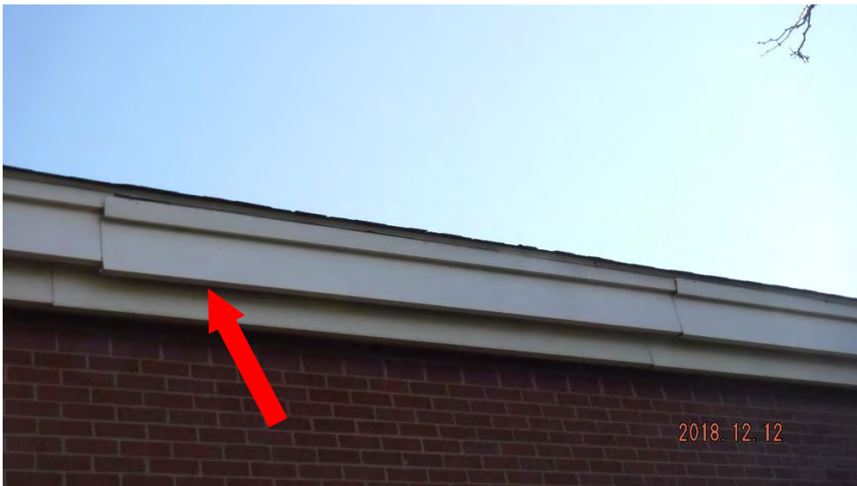
4b. Unsecured/loose fascia metal (see #4 on elevation photo for location).
