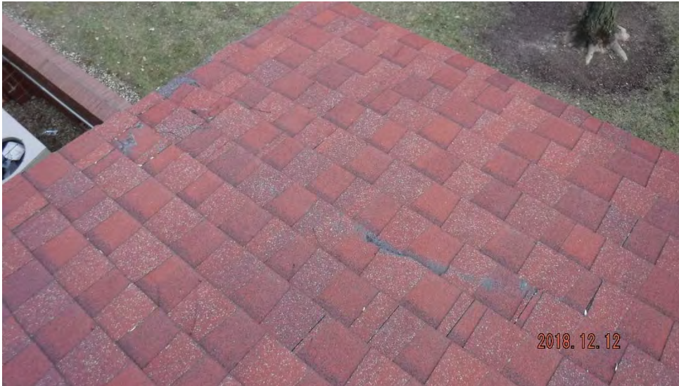
3a. Damaged shingle area (see #3 on plan view for location).
