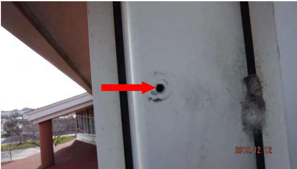
2a. Hole in steel member where item was removed (see #2 on plan view for location).
