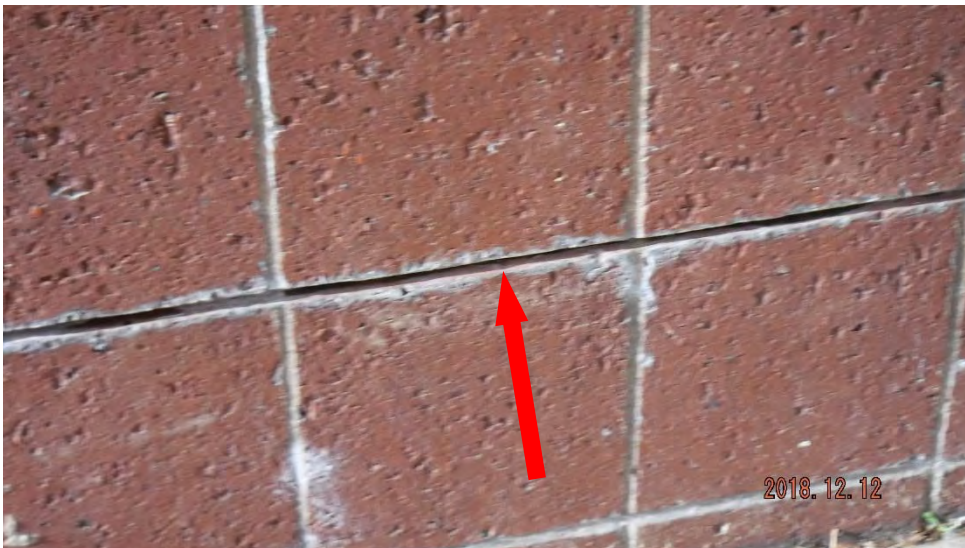
1b. Missing mortar at masonry joint (see #1 on elevation photo for typical location).
