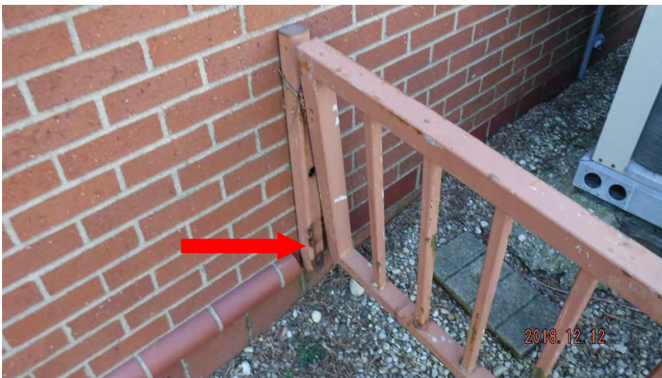
6a. Broken gate hinge (see #6 on elevation photo for location)
