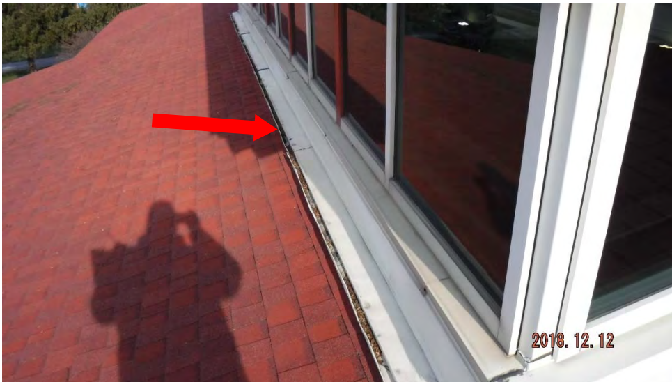
2a. Overview of headwall vent at clerestory (see #2 on plan view for location).
