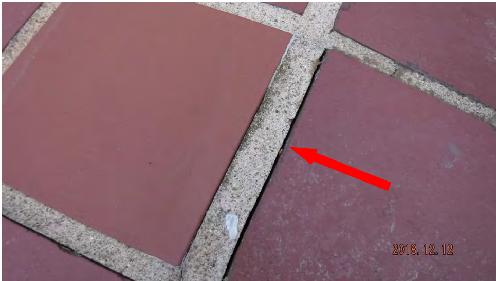
1d. Cracked/shrunk mortar joint(s) (see #1 on elevation photo for typical location).
