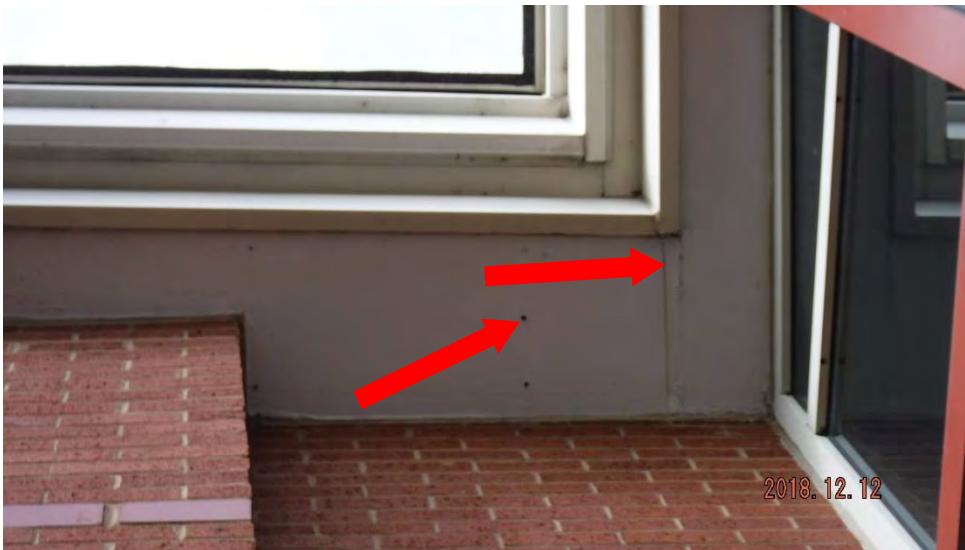
4b. Exposed fasteners and cracked joint (see #4 on elevation photo for typical location).
