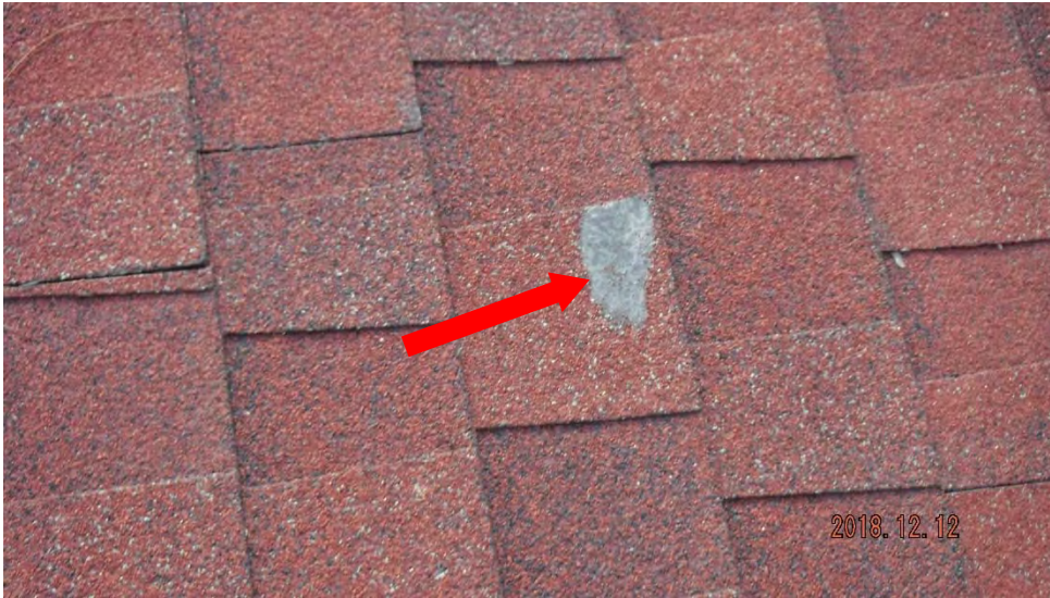
3b. Exposed fabric in deficient shingle (see #3 on plan view for typical locations).
