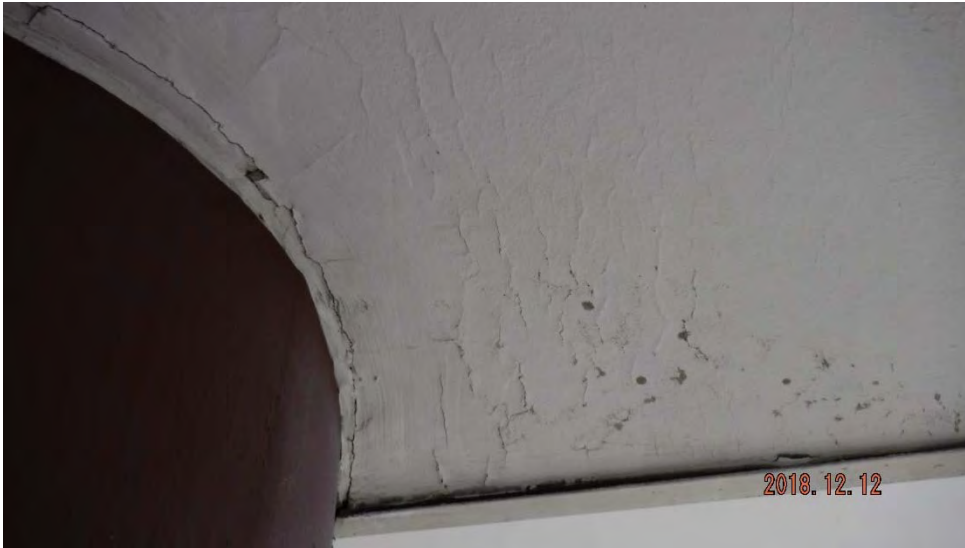
2e. Deterioration of soffit ceiling and chipping/flaking paint (see #2 on elevation photo for typical location).
