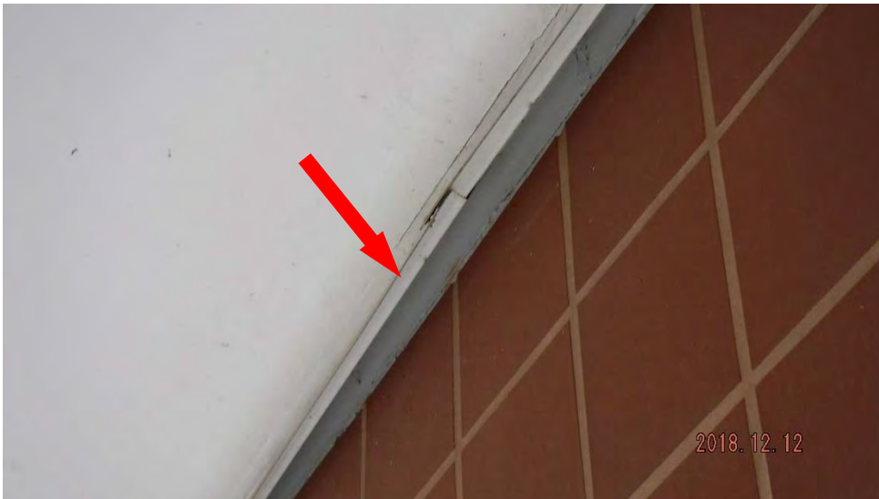
2j. Missing metal flashing (see #2 on elevation photo for typical location).
