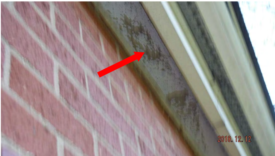
2b. Chipping/flaking paint (see #2 on elevation photo for typical location).
