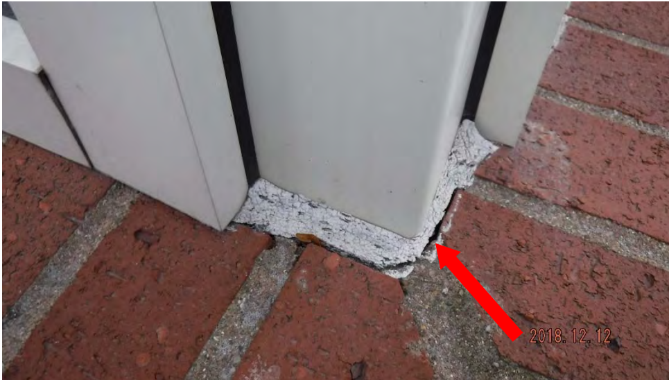
1a. Cracking/shrunk sealant joints (see #1 on elevation photo for location).
