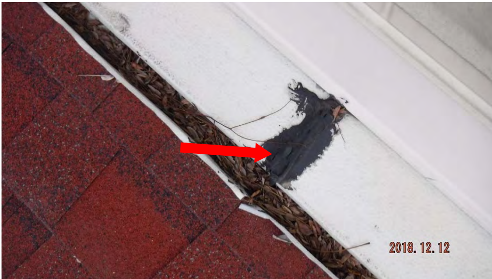
2c. Cracking of the sealant at the vent joint (see #2 on plan view for typical location).
