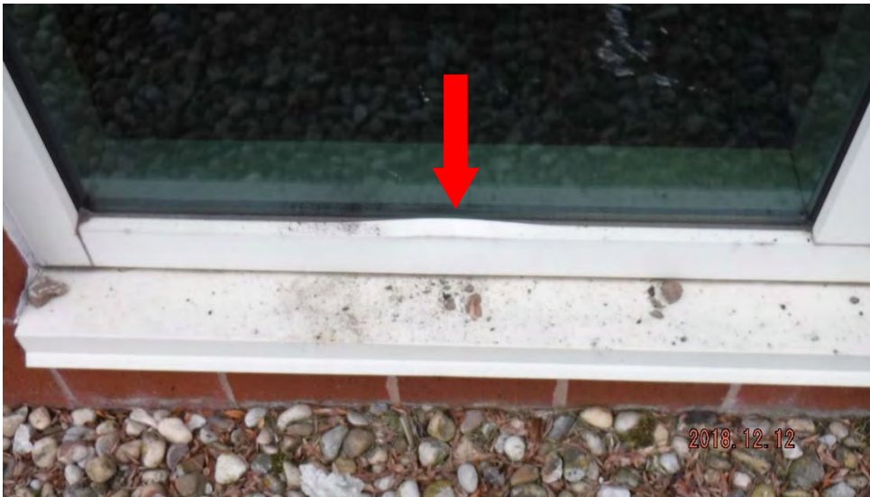
5a. Damage to window pressure plate (see #5 on elevation photo for location).
