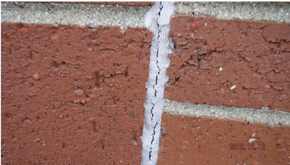
4a. Cracked/shrunk masonry control sealant joint (see #4 on elevation photo for location).
