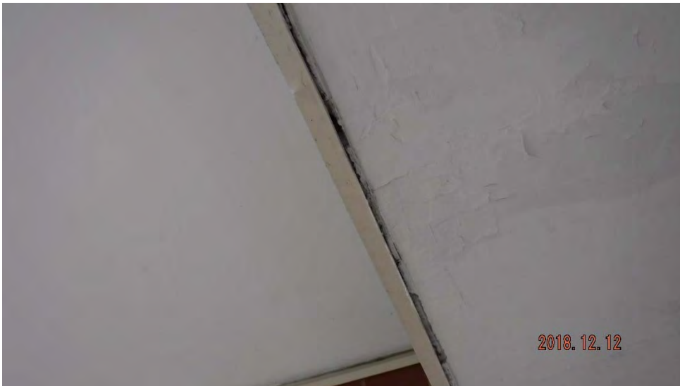
2f. Deterioration of soffit ceiling and chipping/flaking paint (see #2 on elevation photo for typical location).
