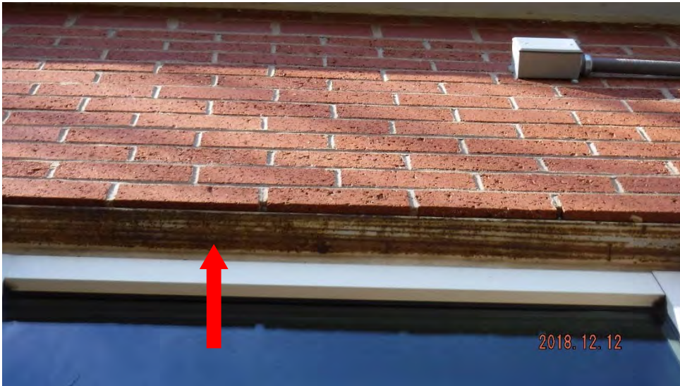
7a. Corrosion on window lintel (see #7 on elevation photo for location).
