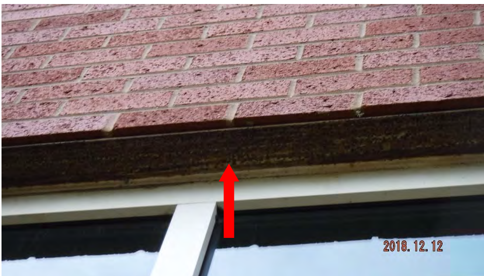
3a. Corrosion on window lintel (see #3 on elevation photo for location).
