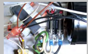
Transformer and fuses.
